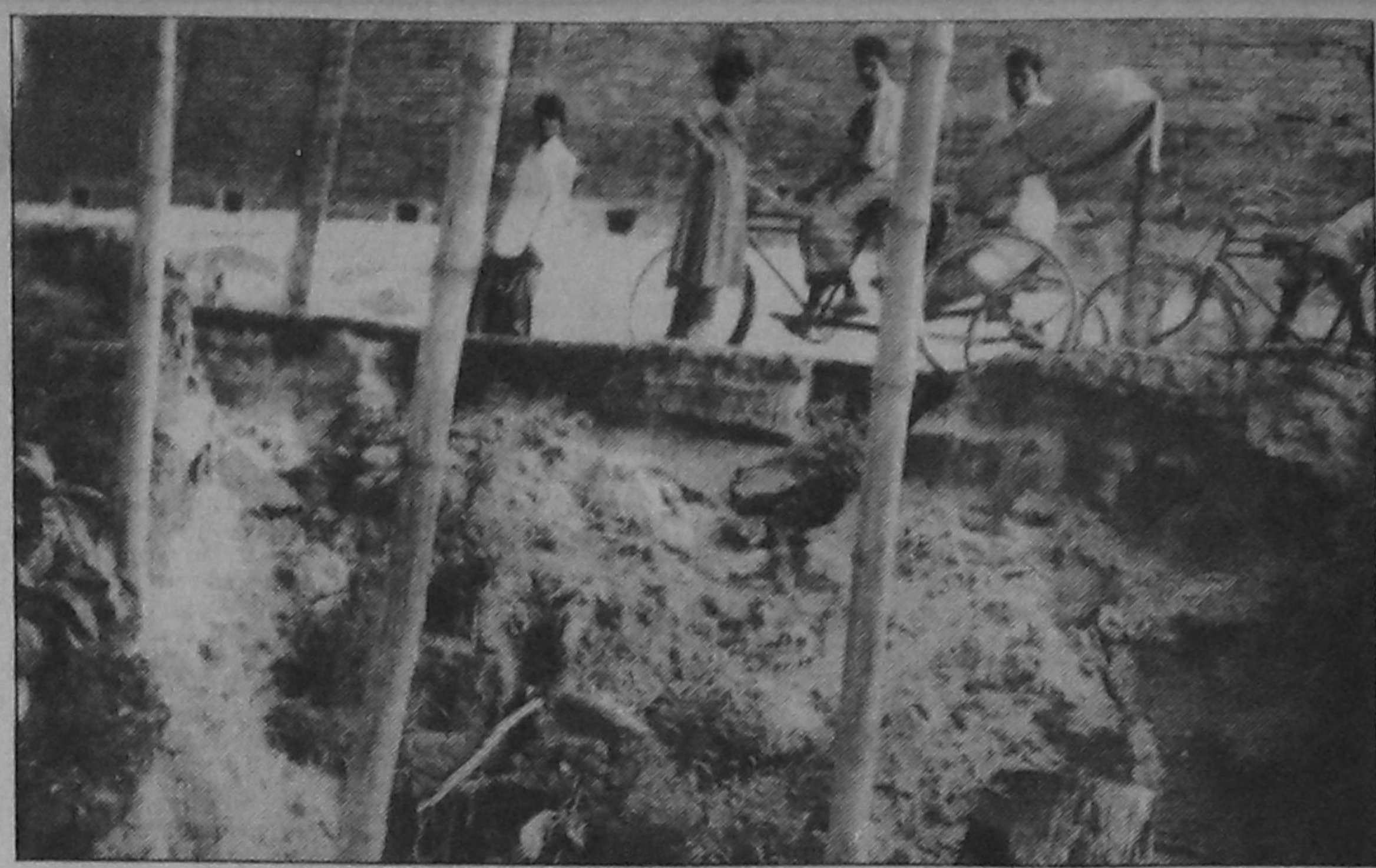
A newly constructed road in Bazaar Station area in Sirajganj town collapses recently. Local people allege substandard construction materials were used in the road. — Star photo
