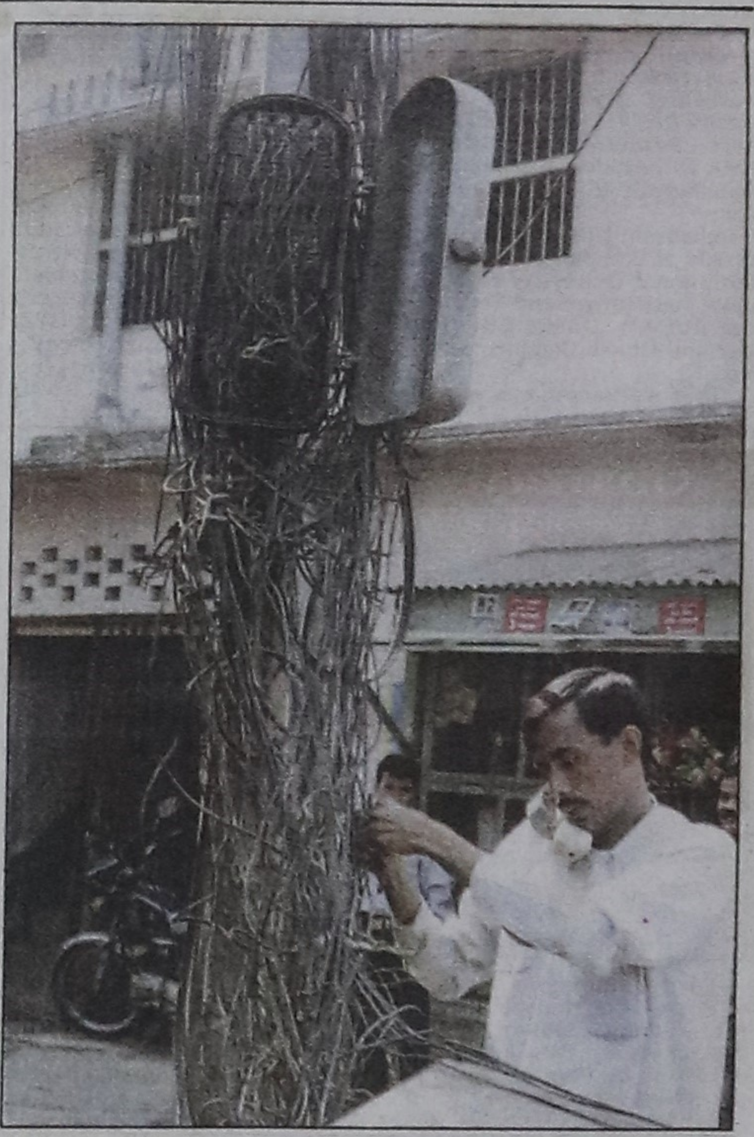
Telecom tangle. Tightly tangled telephone cables at a business hub in Narayanganj poignantly speak of the state of affairs in Bangladesh. Star photo: A K M Mohsin
