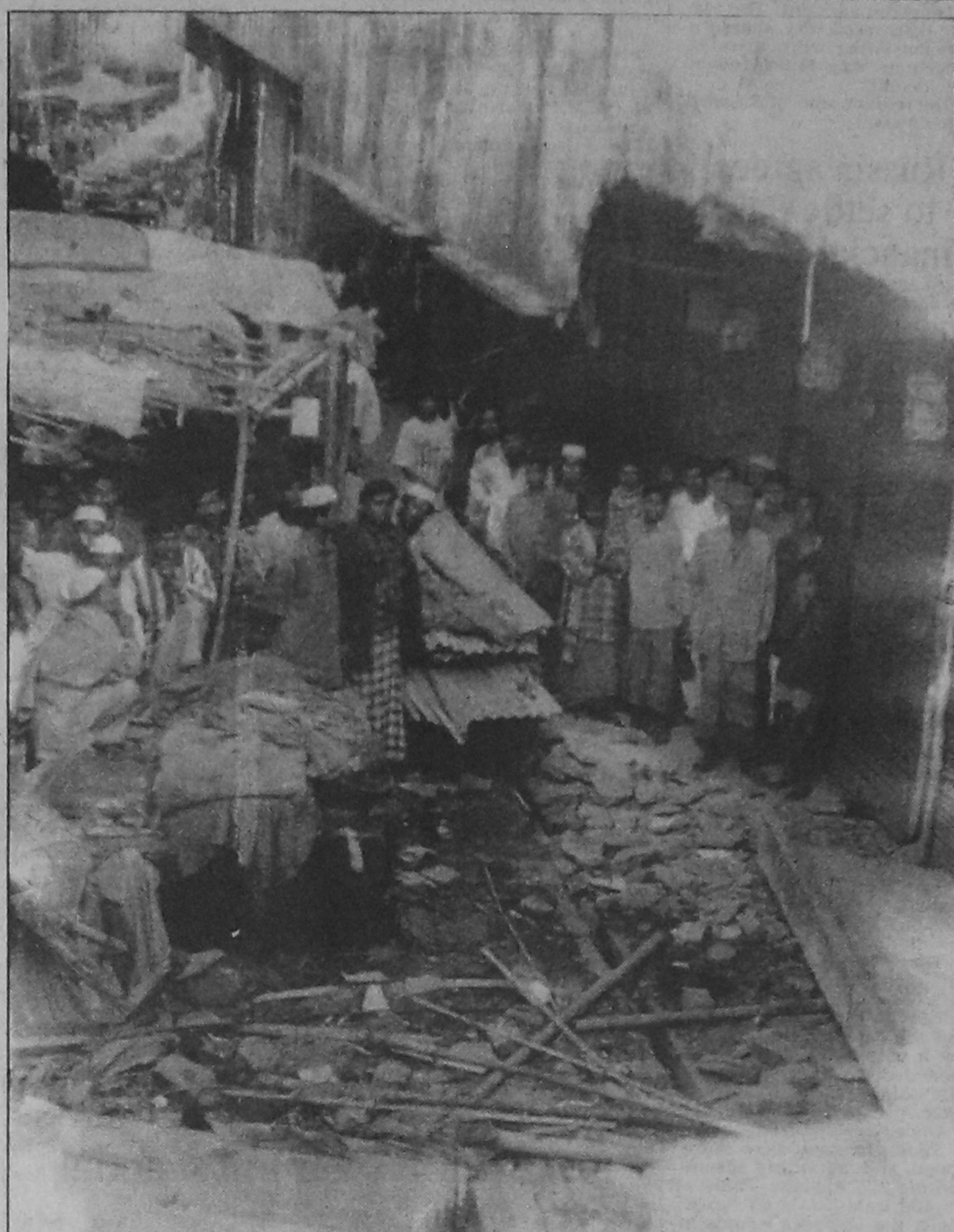
An under-construction building collapsed at Rayer Bazar in the city injuring five people yesterday.
