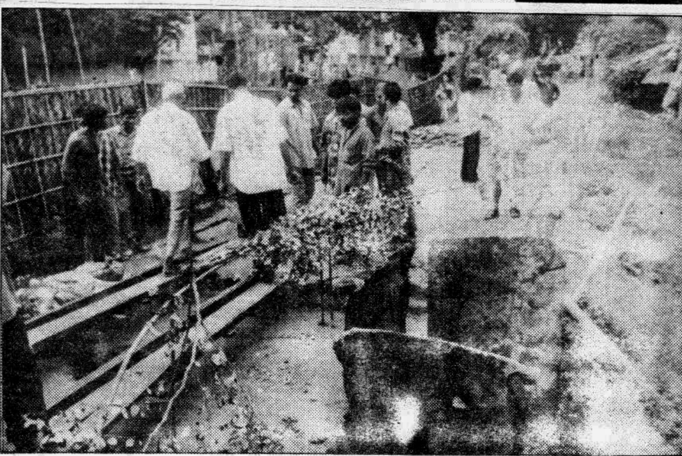
Heavy rainfall during Tuesday night has left the makeshift road on the lake at Dhanmondi Road No 32 on the verge of collapse. Wooden planks have been placed there to ease movement by pedestrians. — Star photo
