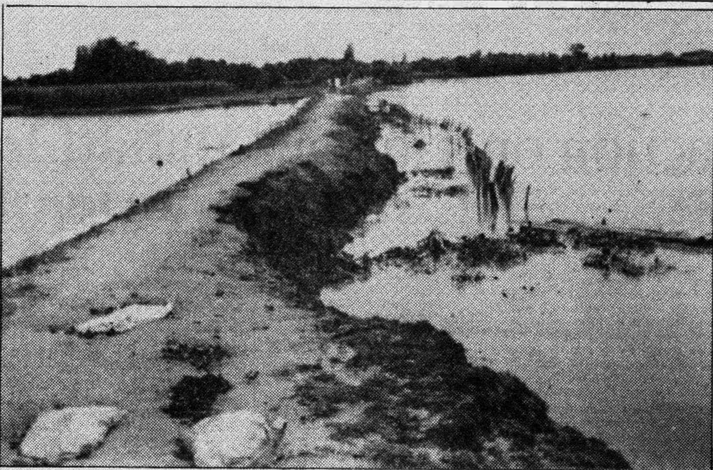
Flood damaged Bochadhaha embankment at Mohimaganj in Gobindaganj thana of Gaibandha district. — Star photo
