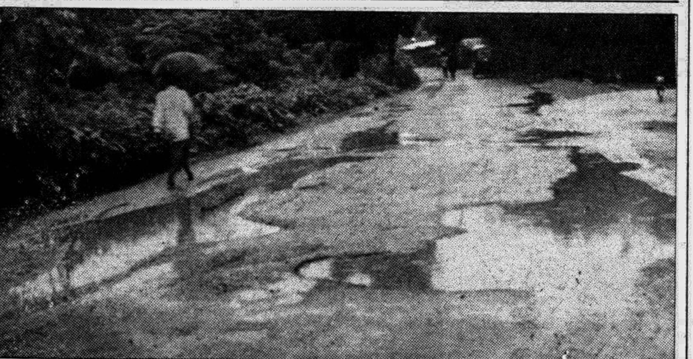
Innumerable cracks and potholes have been developed on Saikupa-Garaganj highway in Jhenidah district making it quite unfit for use. Yet vehicles are plying unabated on this highway resulting in untold sufferings to hundreds of passengers. — Star photo
