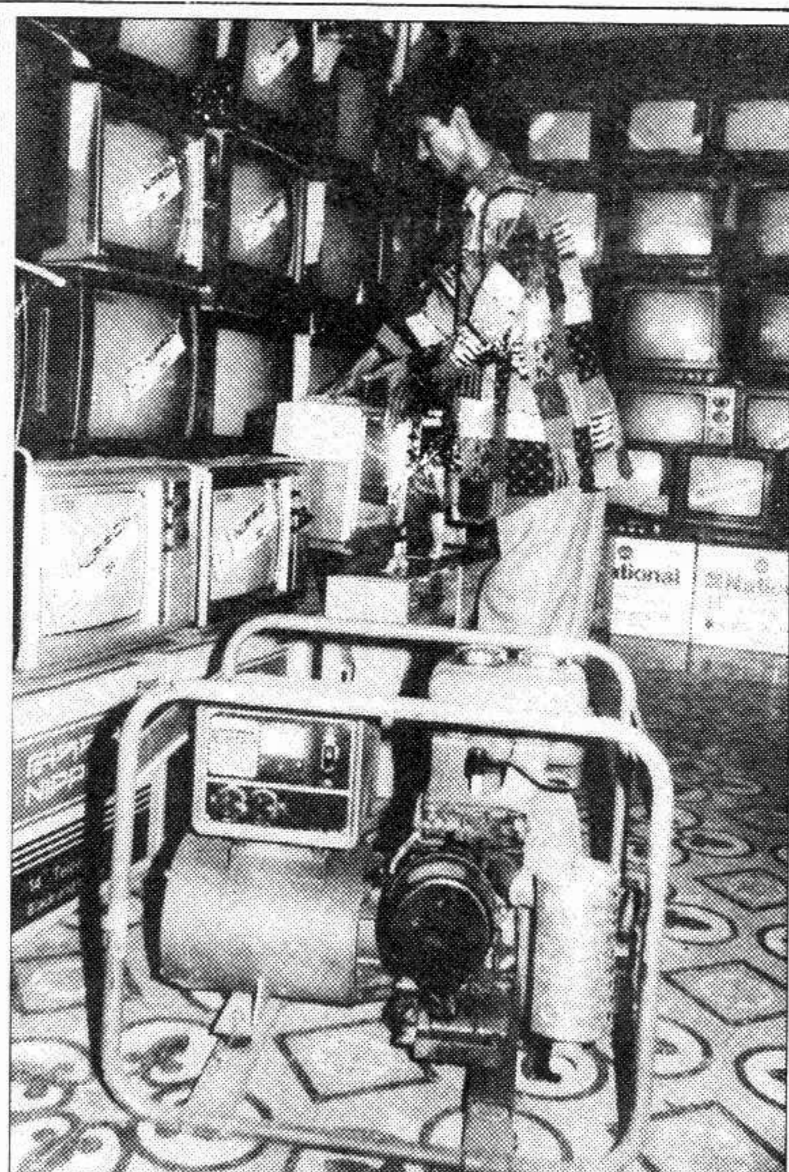
To cope with the unprecedented load-shedding of electricity now prevailing in the city, the shopowners in different markets are busy installing generators in their business establishments. This picture was taken yesterday from the Baitul Mukarram Electronics Market. — Star photo
