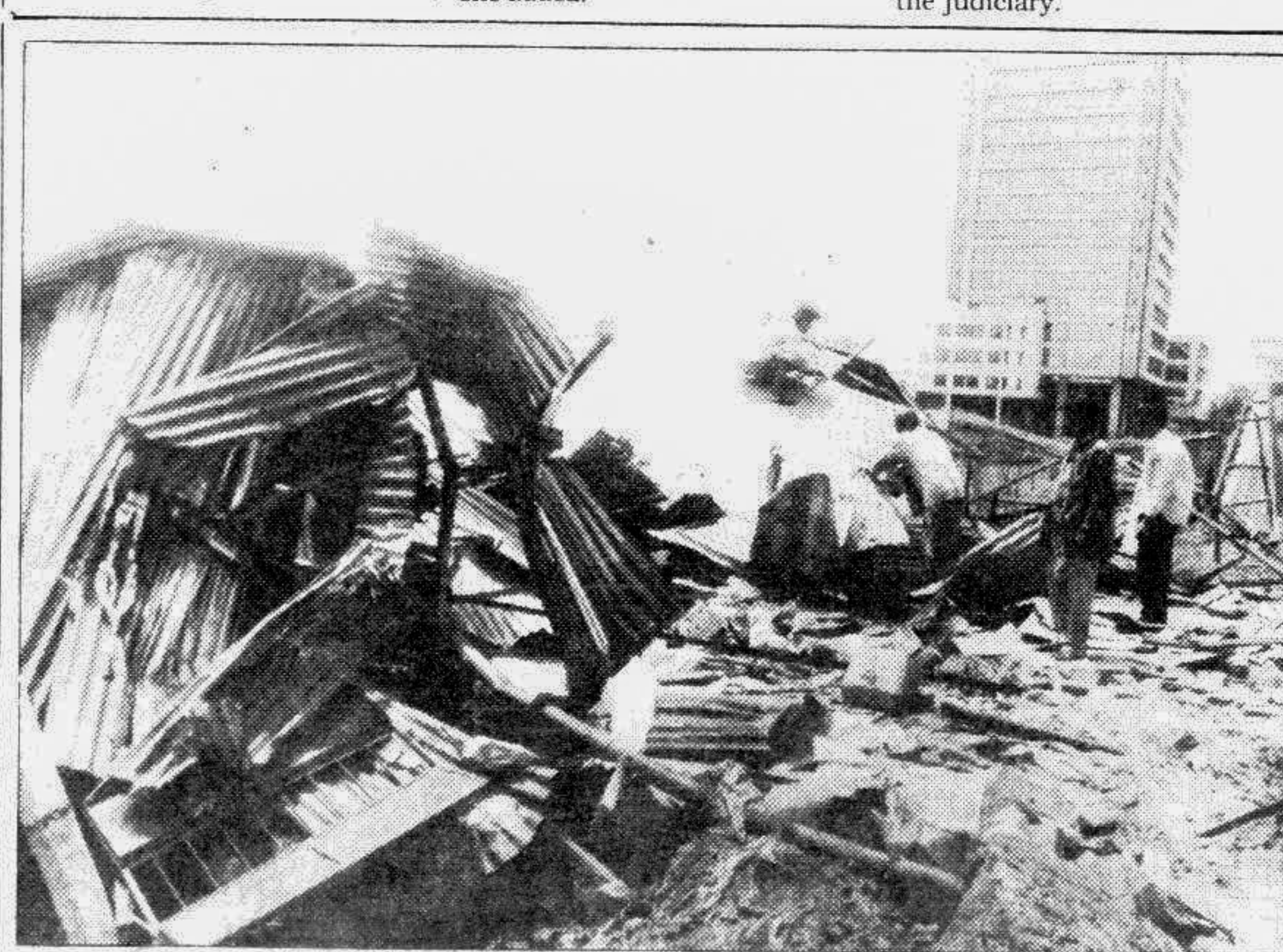
Rajuk drive underway yesterday to demolish unauthorised structures near the lake at Gulshan Section-I in the city. — Star photo
