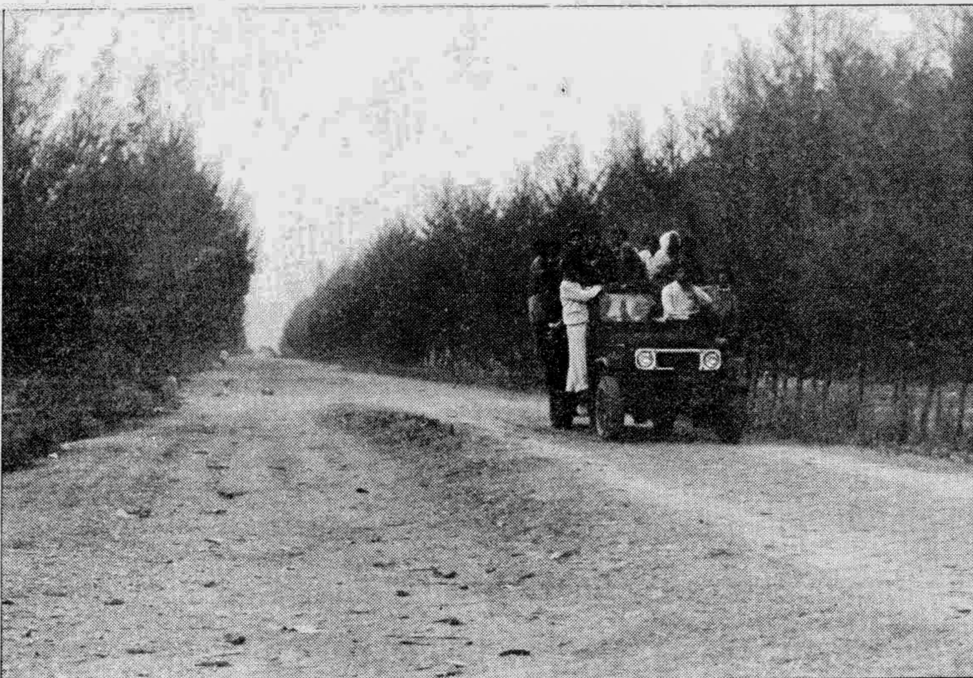
COX'S BAZAR: A new road along Cox's Bazar-Teknaf sea beach is now under construction for the recreation of tourists from home and abroad. — Star photo by A K M Mohsin
