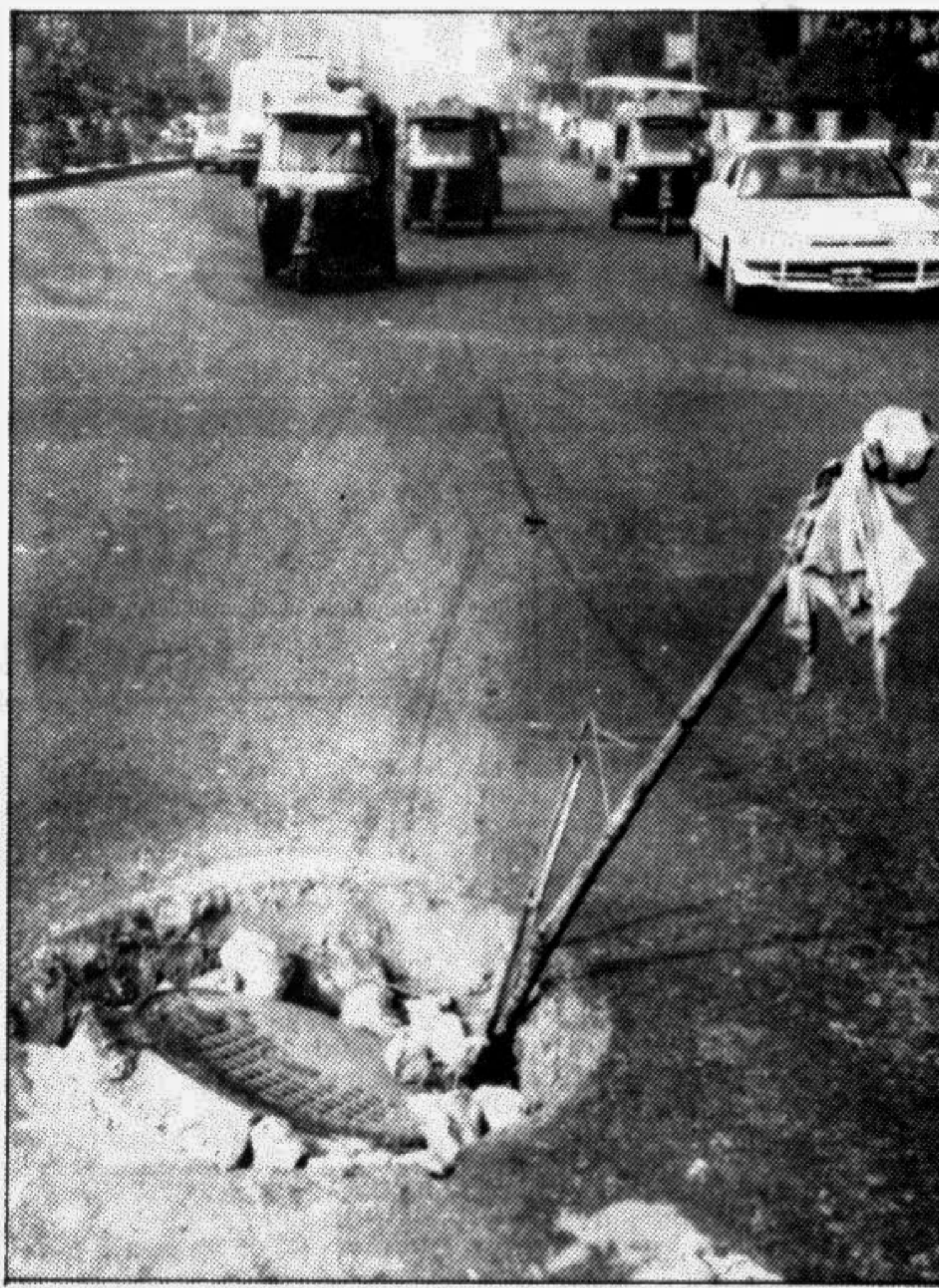
A dilapidated manhole cover on the VIP road near Dhaka Sheraton Hotel posing a real threat to pedestrians as well as vehicular movement. — Star photo
