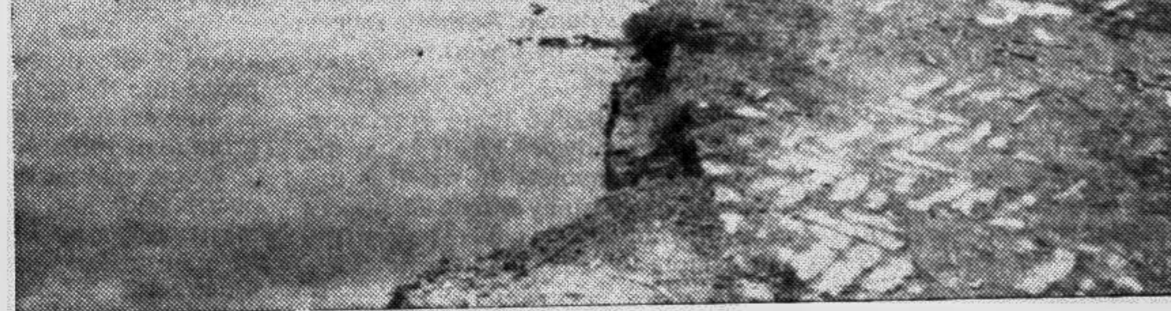
PABNA: Floods have damaged very badly Buddhaerhat Road of Bablatala situated under Pabna Pourashava. — Star photo
