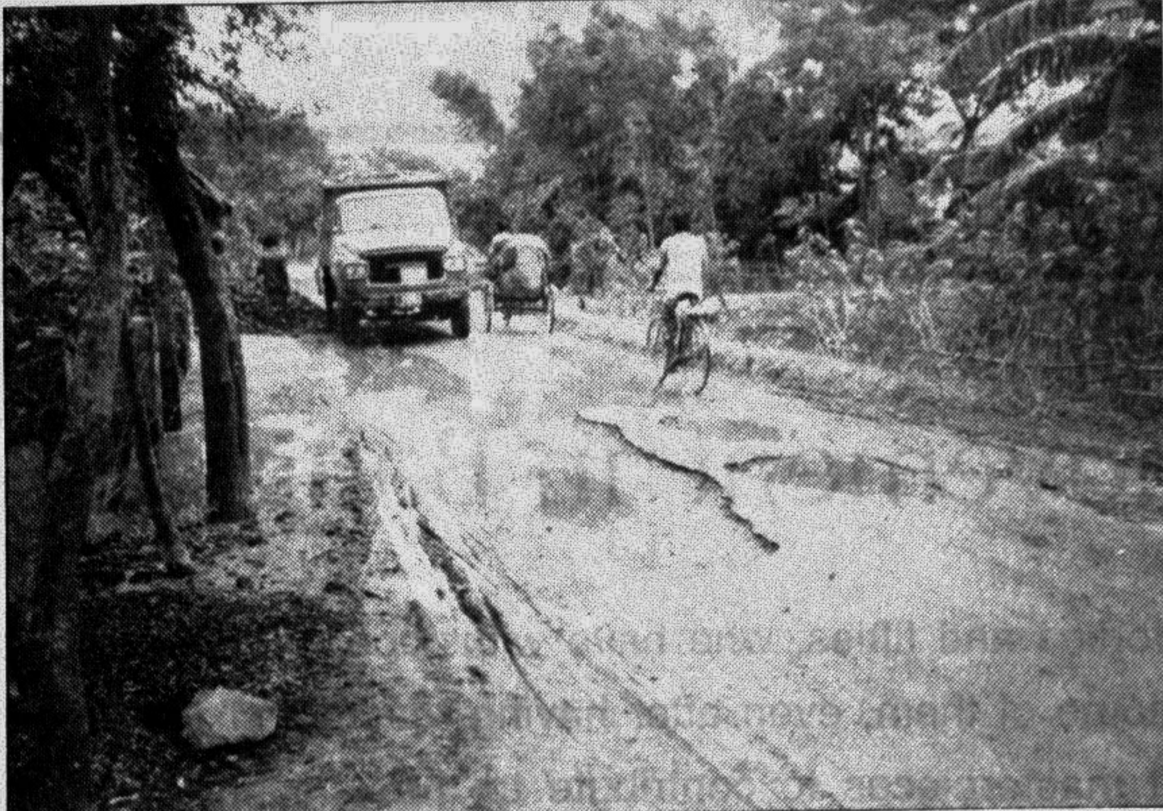
GAIBANDHA: Fund shortage hampering the repair work of flood damaged Gaibandha-Sadullapur road. — Star photo
