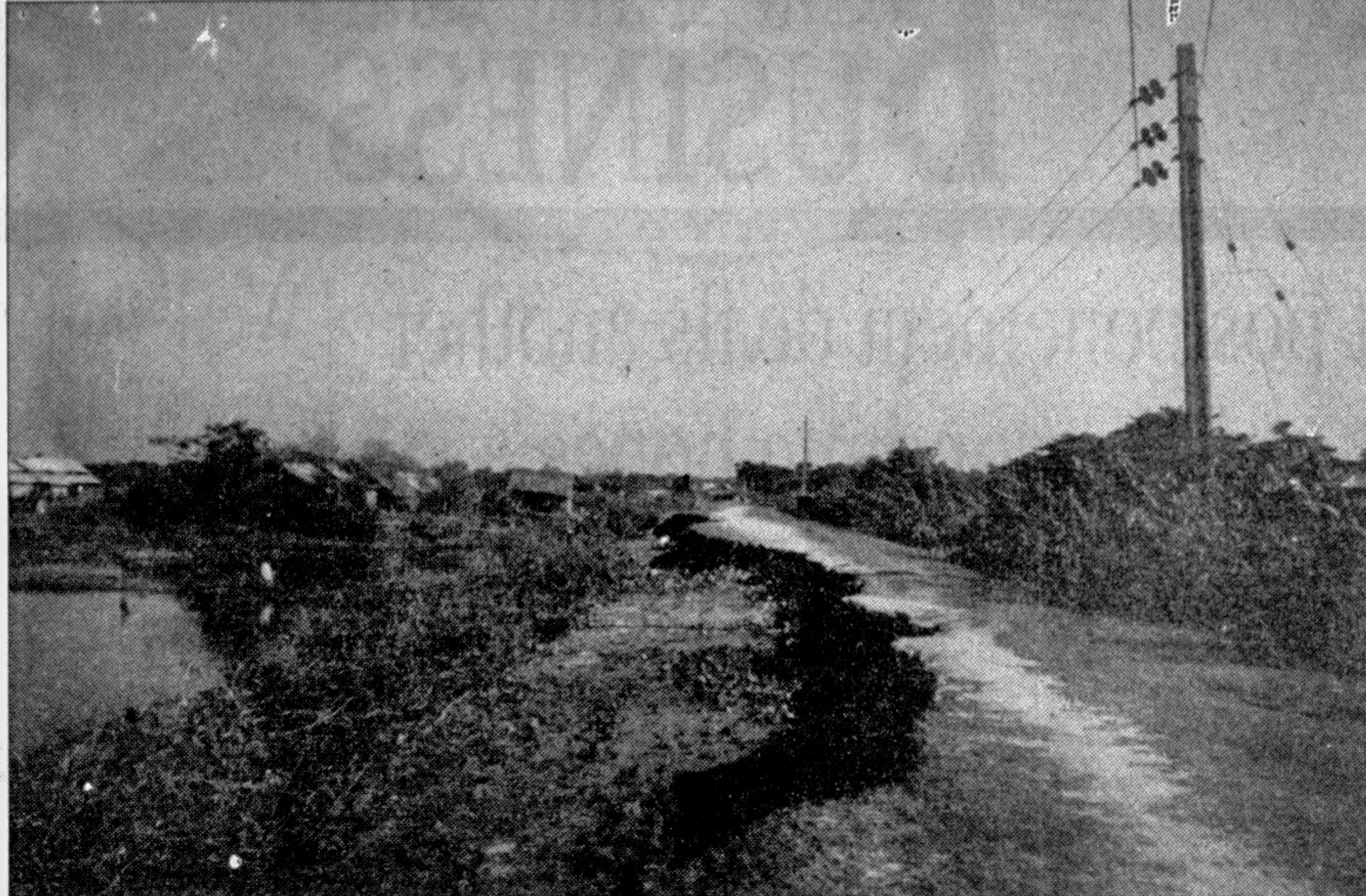
SYLHET: Jagannathpur-Chilaura road in Sunamganj district has been badly damaged by the recent floods. A good portion of the road measuring about five kilometres has been washed away. — Star photo
