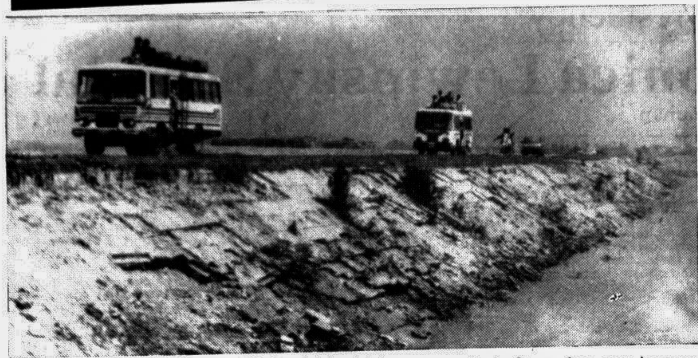
DANGER OUT THERE: The Dhaka-Aricha highway near Amin Bazar has now become risky for the traffic as flood waters eroded edges of either side of the road. — Star photo
