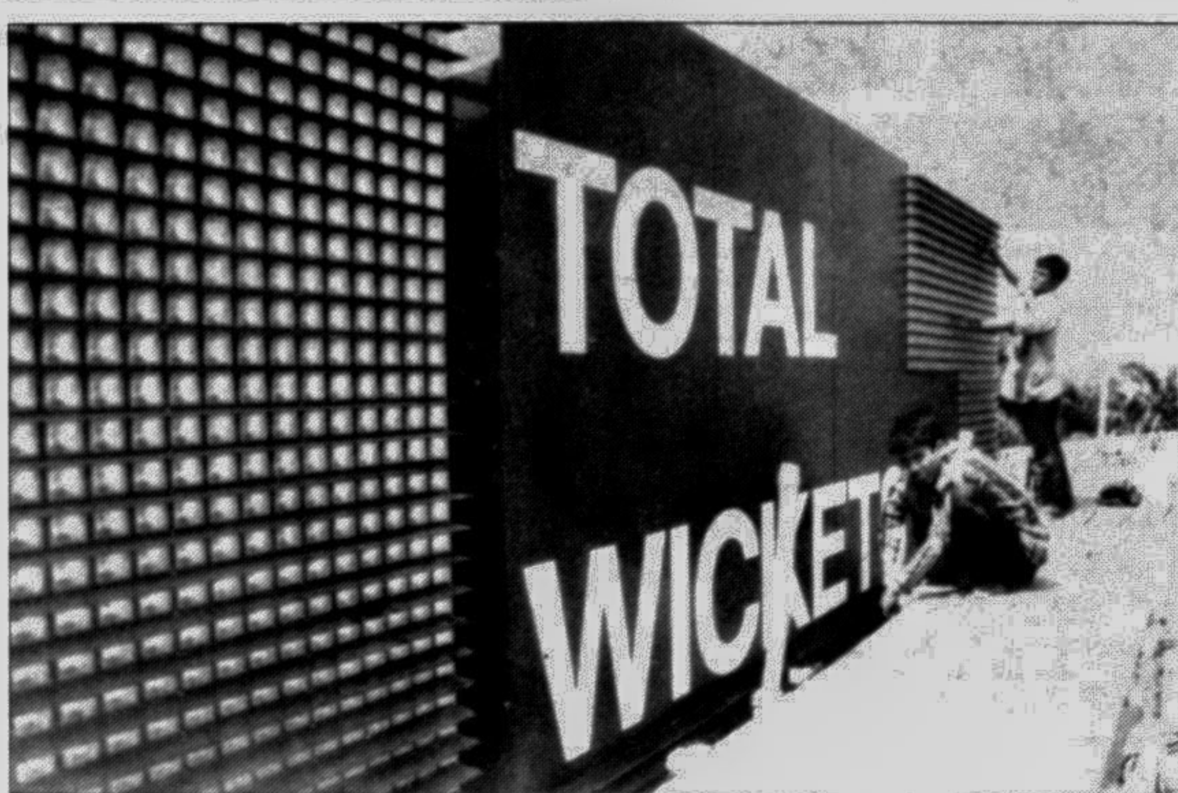
The 30 million-taka electronic scoreboard is in the final stages of erection at the Bangabandhu Stadium. The formal inauguration will be held on 12 October.
