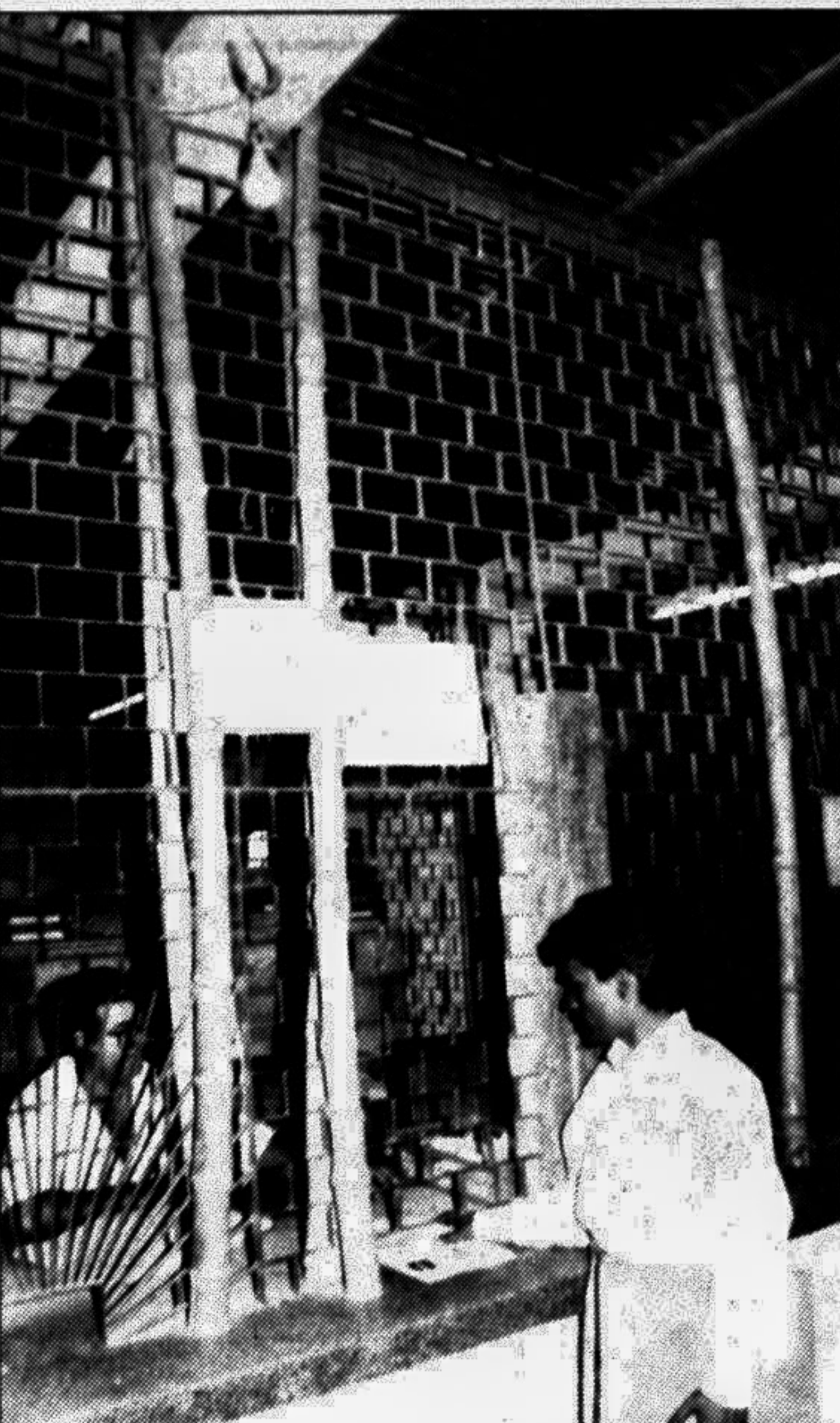
Makeshift arrangement has been made to ward off the threat posed by the worn-out roof of Certificate Section of the DU's administrative building. — Star photo
