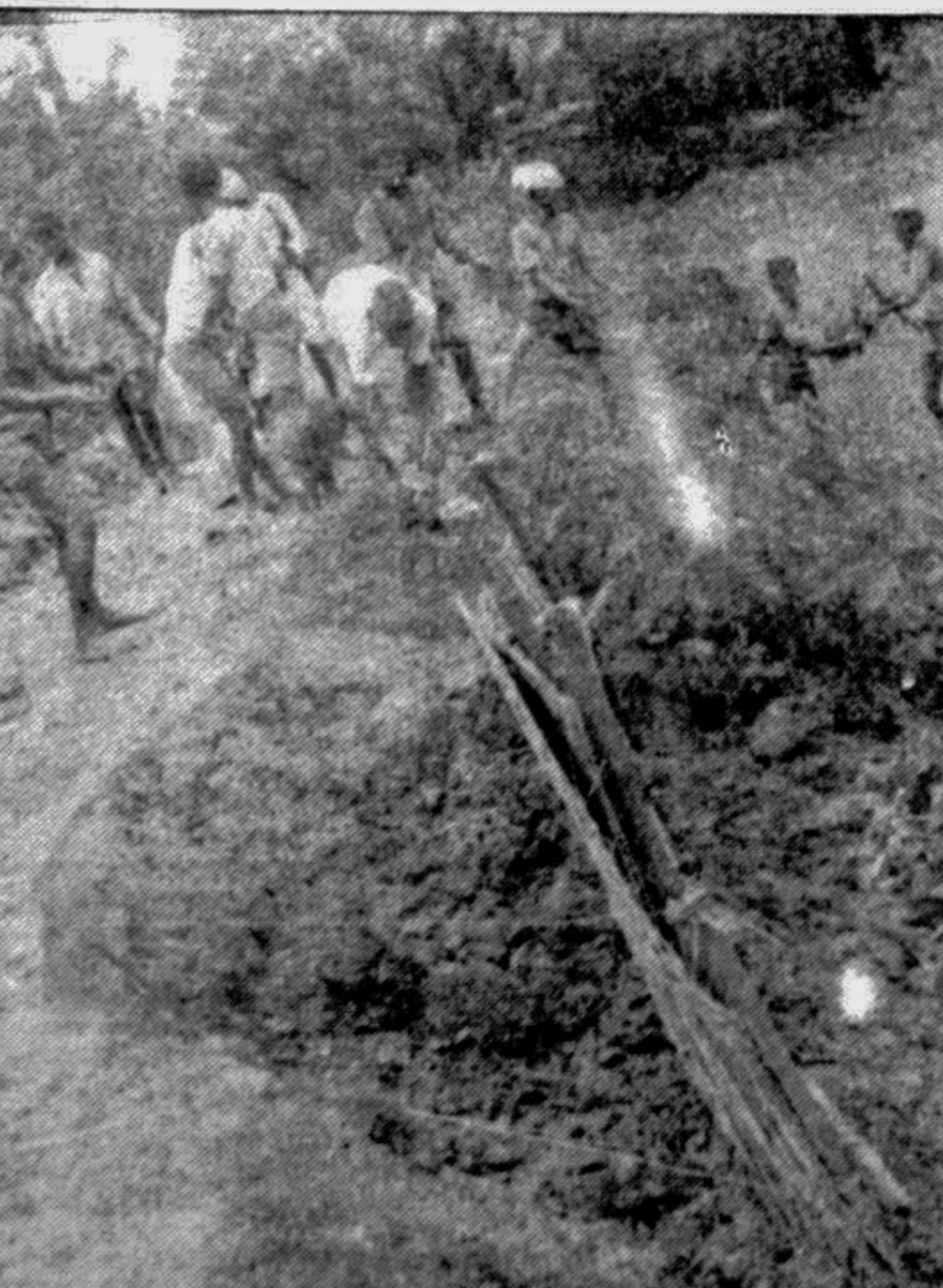
NOAKHALI: Local villagers recently worked round-the-clock to repair the dam of Kaluai Multipurpose Rupali Irrigation project which was affected by flood. The project covers 300 acres of land at village Kaluai in Number 2 Nadona union of Begumganj thana.
