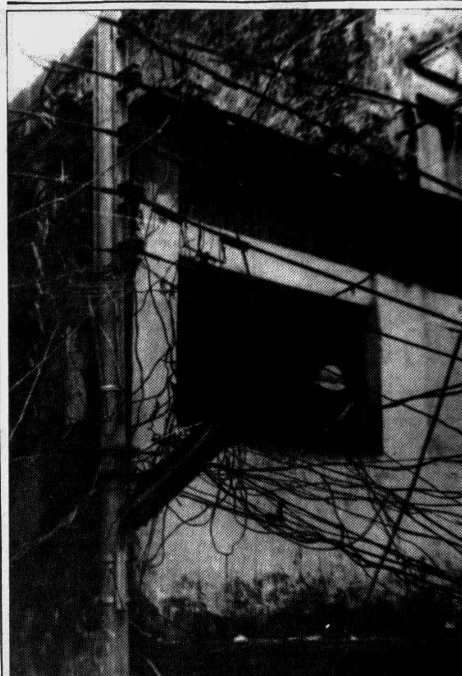
You can call it 'weird wires'. Just imagine, what happens if a fire breaks out, accidentally? — Star photo
