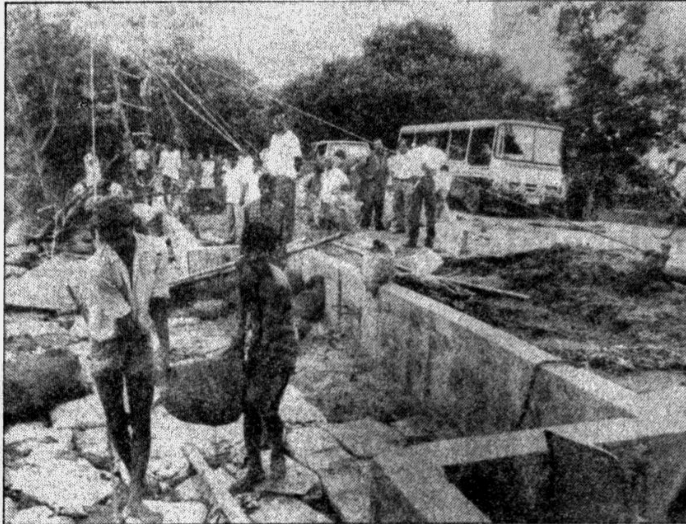
LEAVING NO STONE UNTURNED: Stones are real heavy on the Dhaka-Sylhet Highway. At a place called Barabo, under Rugganj thana, landslides stopped traffic. The photo shows poor labourers work hard to clean up the mess while government engineers watch. Yesterday, our photographer Anisur Rahman also saw military engineers lending a hand and reported that the road was in real danger.
