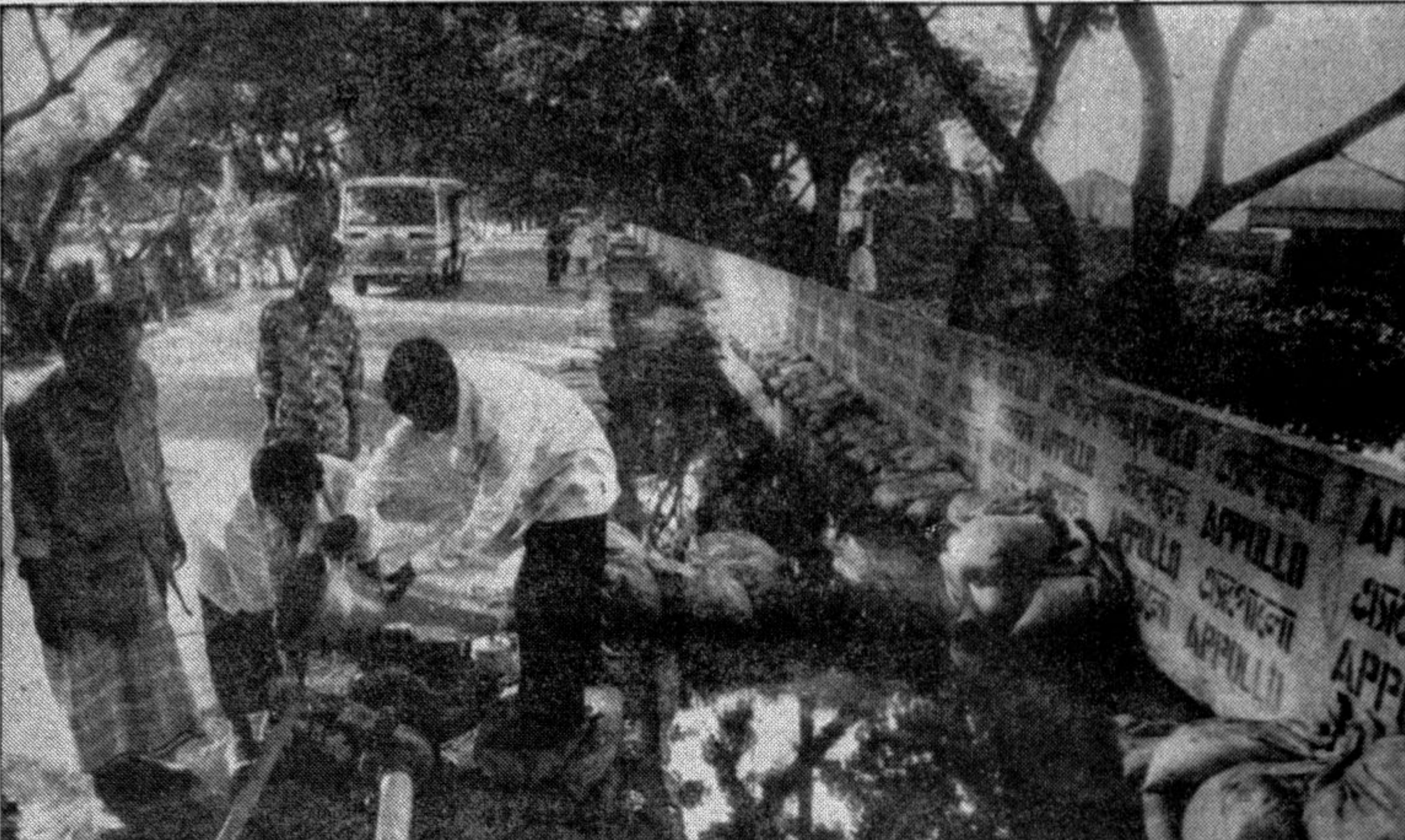
Desperate bid to pump out the water sipping through barrier on to the road (Demra). — Star photo by Amran Hossain
