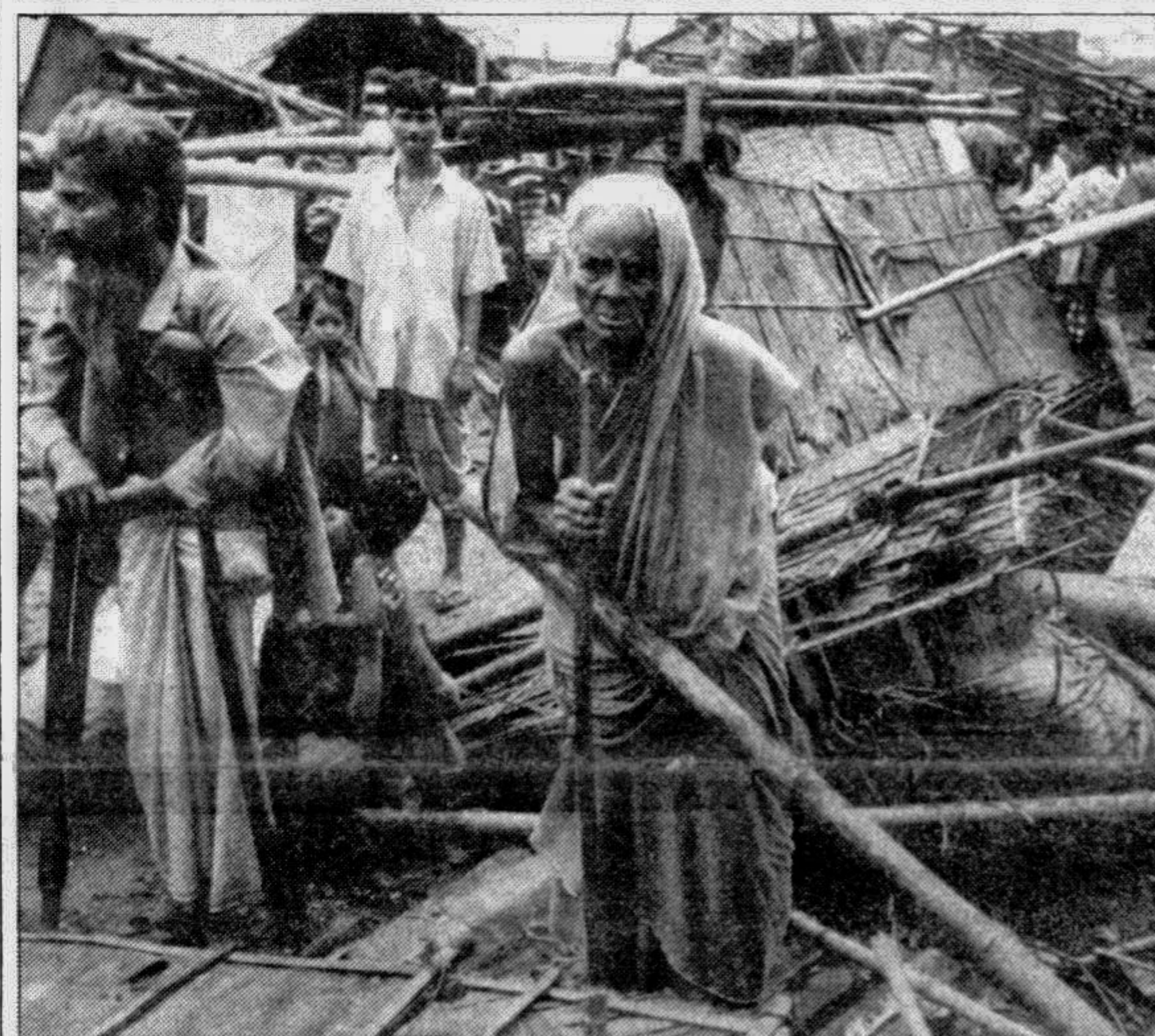
WHAT TO DO NOW: A bewildered old woman and a disabled man standing over the rubbles after their slum near the Sonargaon Hotel was demolished by the Rajuk yesterday.
