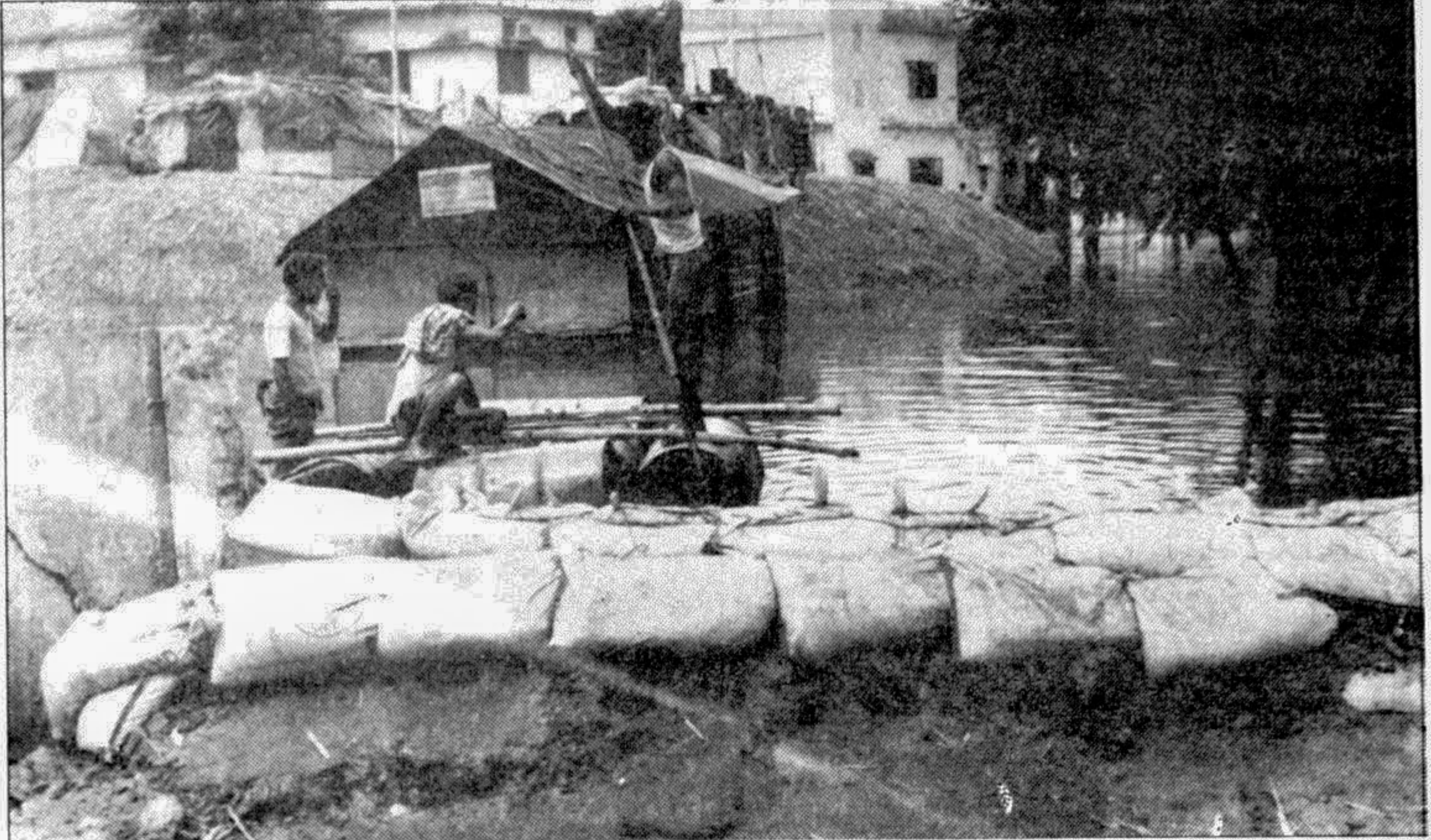
Efforts have been intensified to protect DND embankment from the fury of flood yesterday. — Star photo
