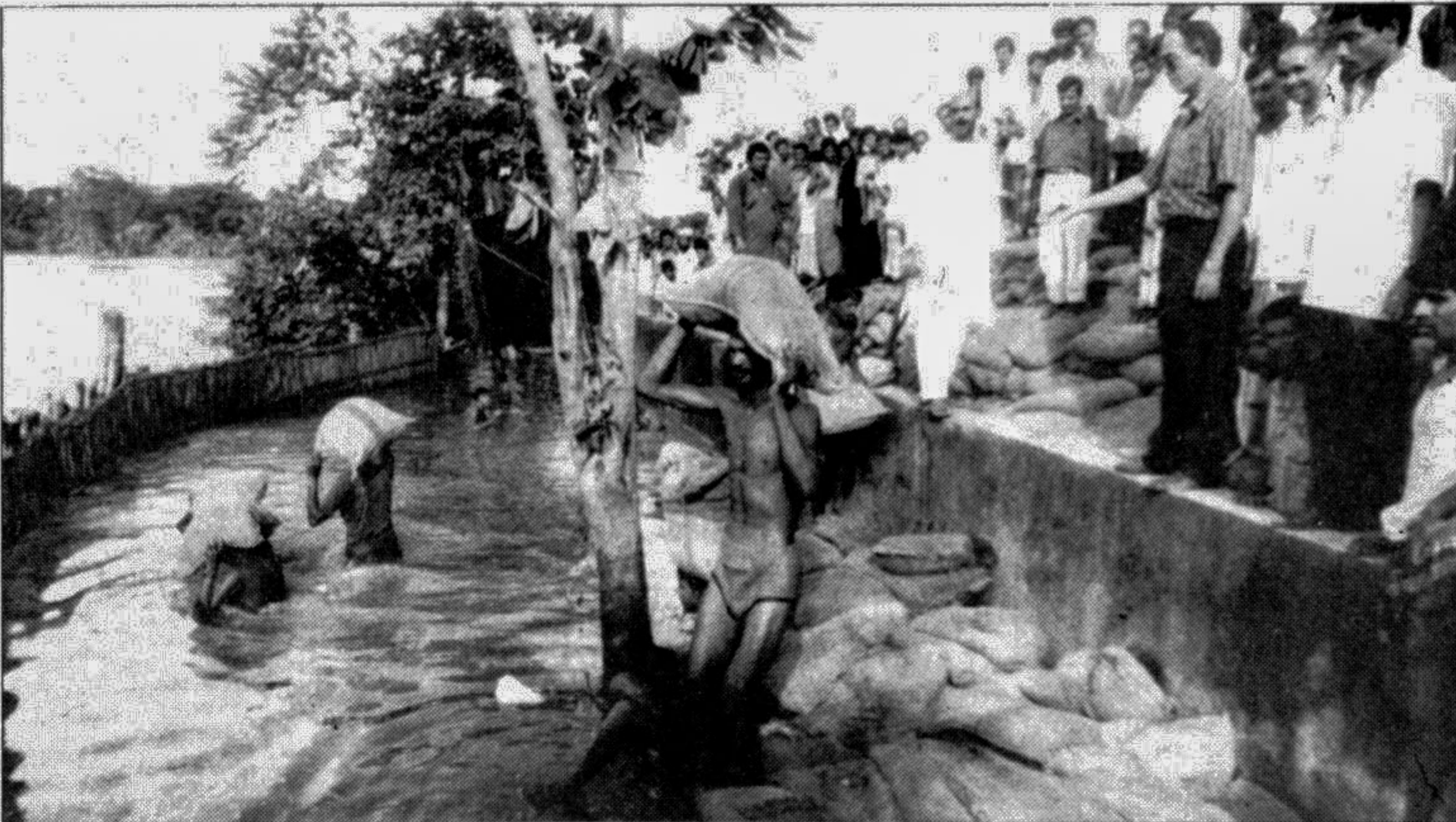
Efforts are underway to save DND embankment threatened by flood waters.
