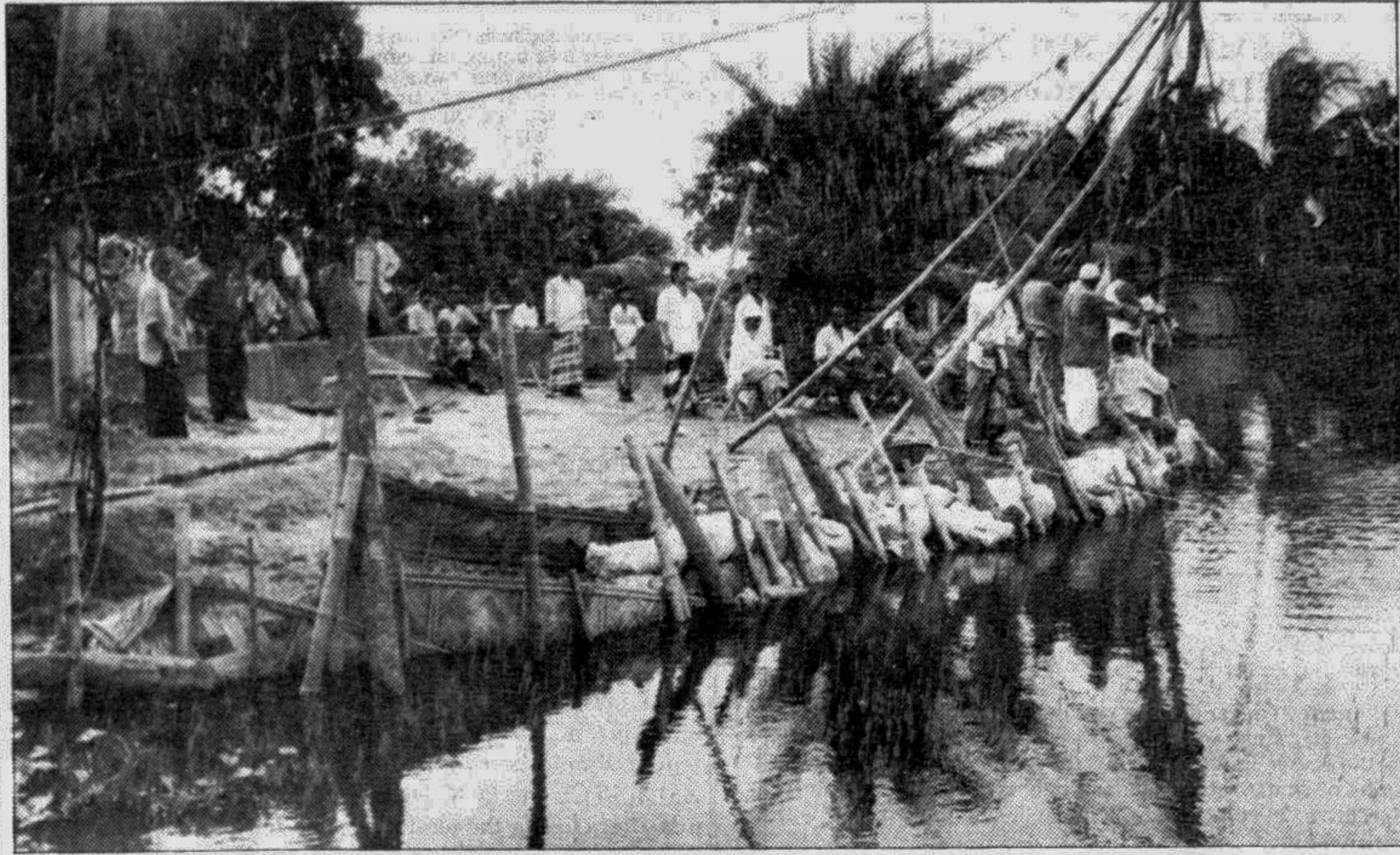
A crack in the DND embankment in the city's Demra area being repaired yesterday. — Star photo
