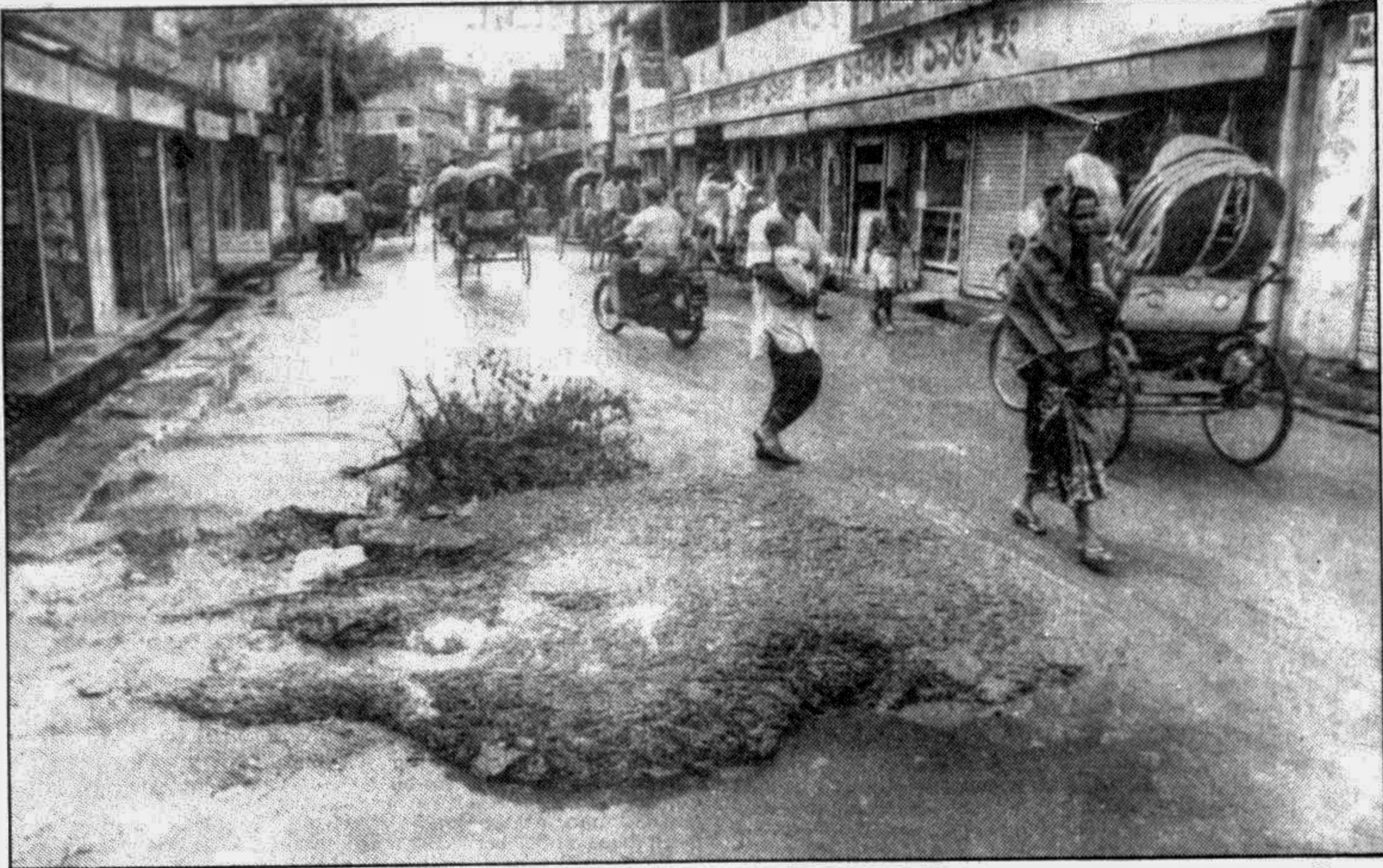
Sewage spilling out of a manhole near Faridabad Madrassah in the city for the last three to four days, polluting the environment, but no action has yet been taken by the authorities concerned to clean the road. — Star photo
