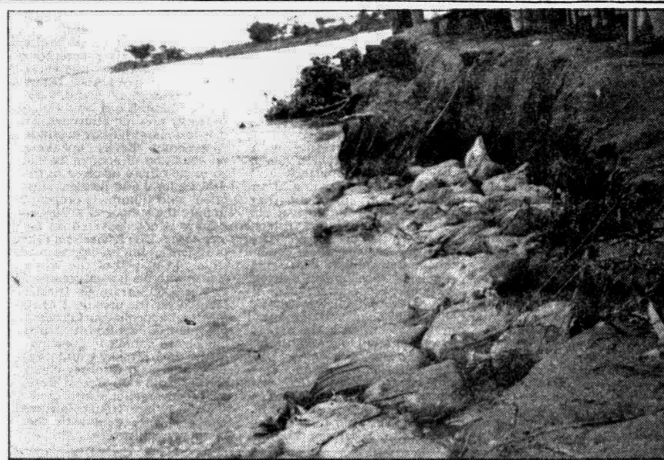
RANGPUR: Erosion of the river Teesta has taken a serious turn in Gangachhara thana despite protective measures taken by the Water Development Board.
