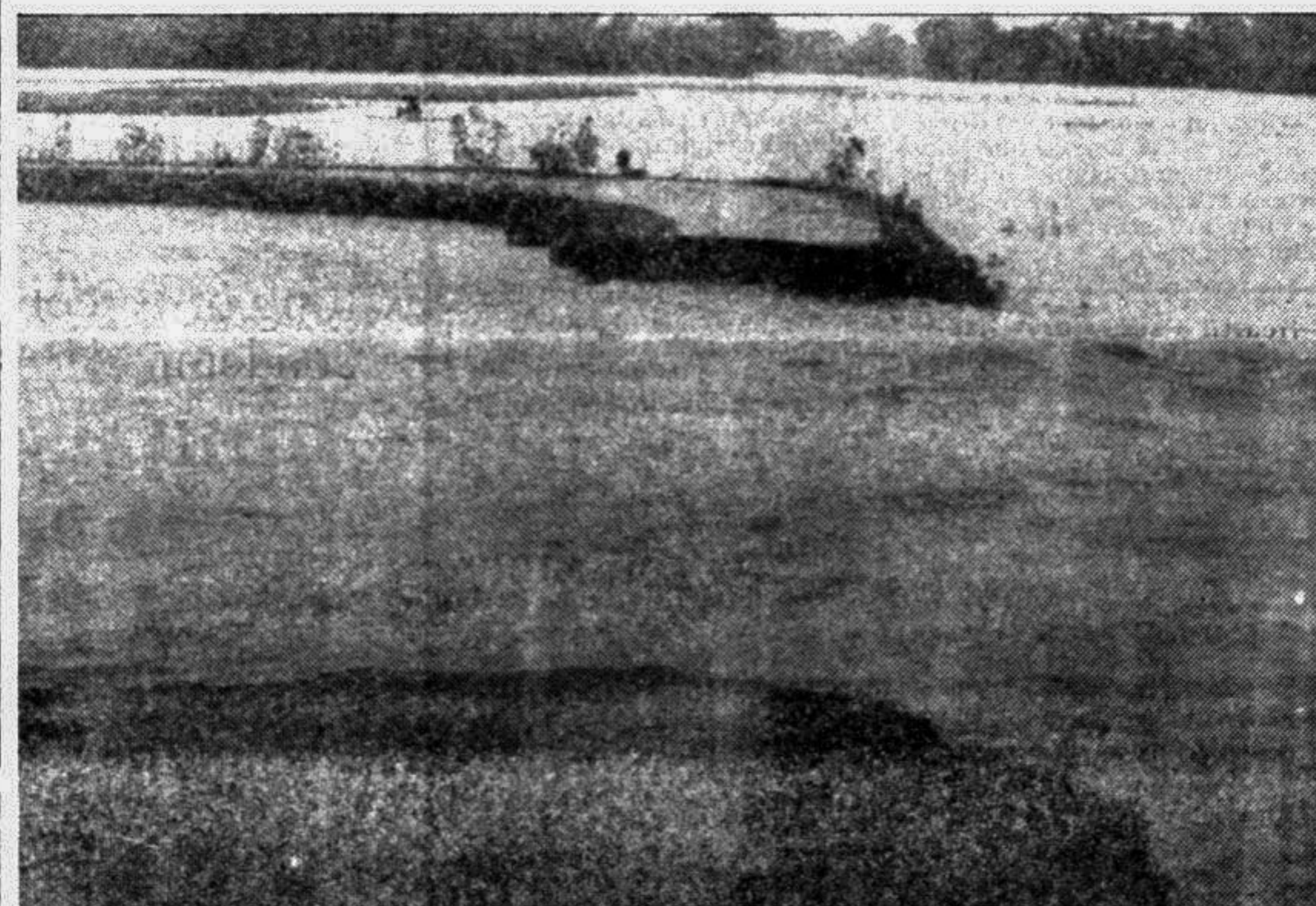
SYLHET: A pucca road at Chankhai Dahar in Golapganj thana has been damaged by gushing water of the river Surma.
