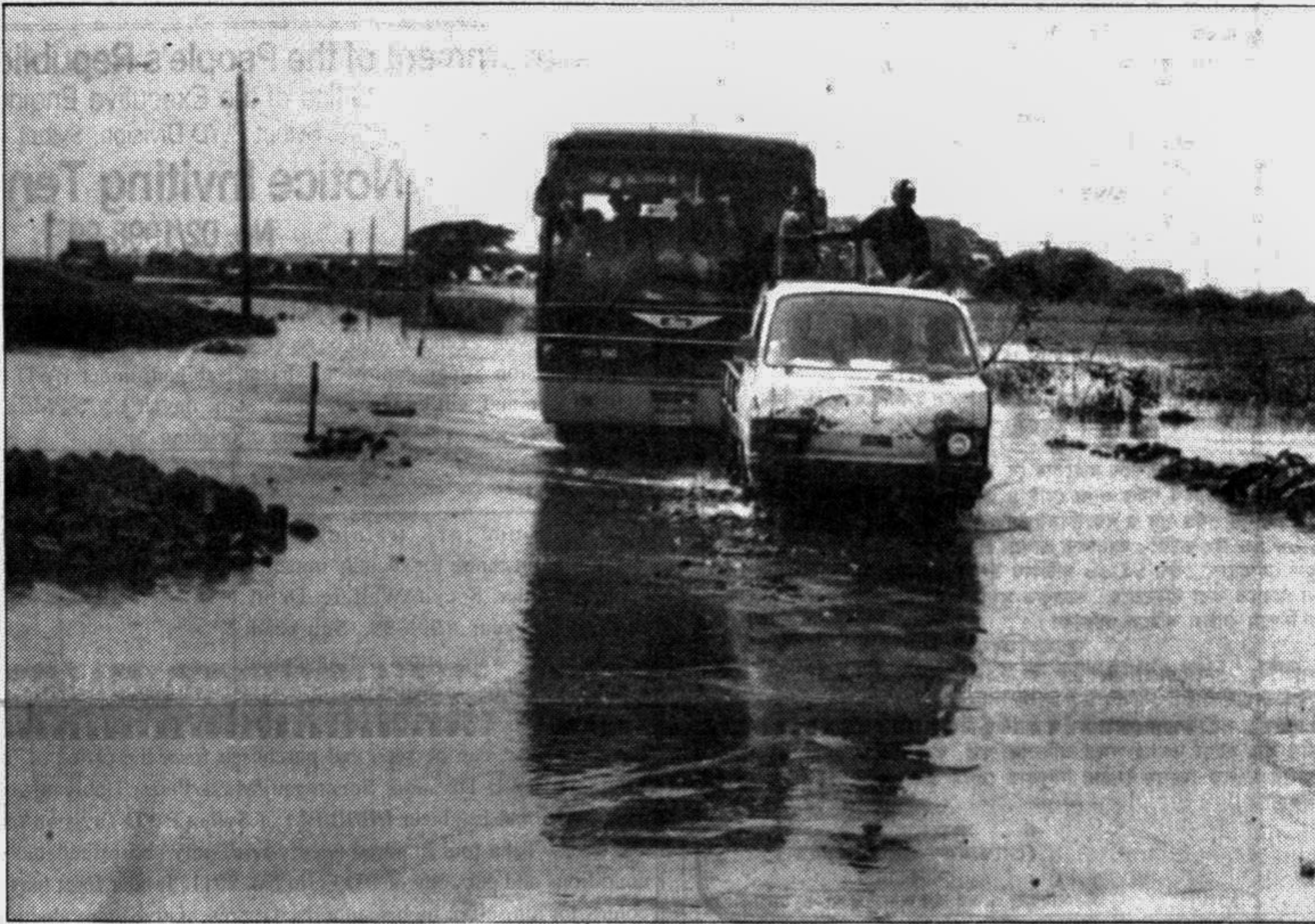
VITAL ROAD-LINK UNDER THREAT: The Dhaka-Chittagong highway at Baniakandi near Meghna Bridge went under flood water yesterday.
