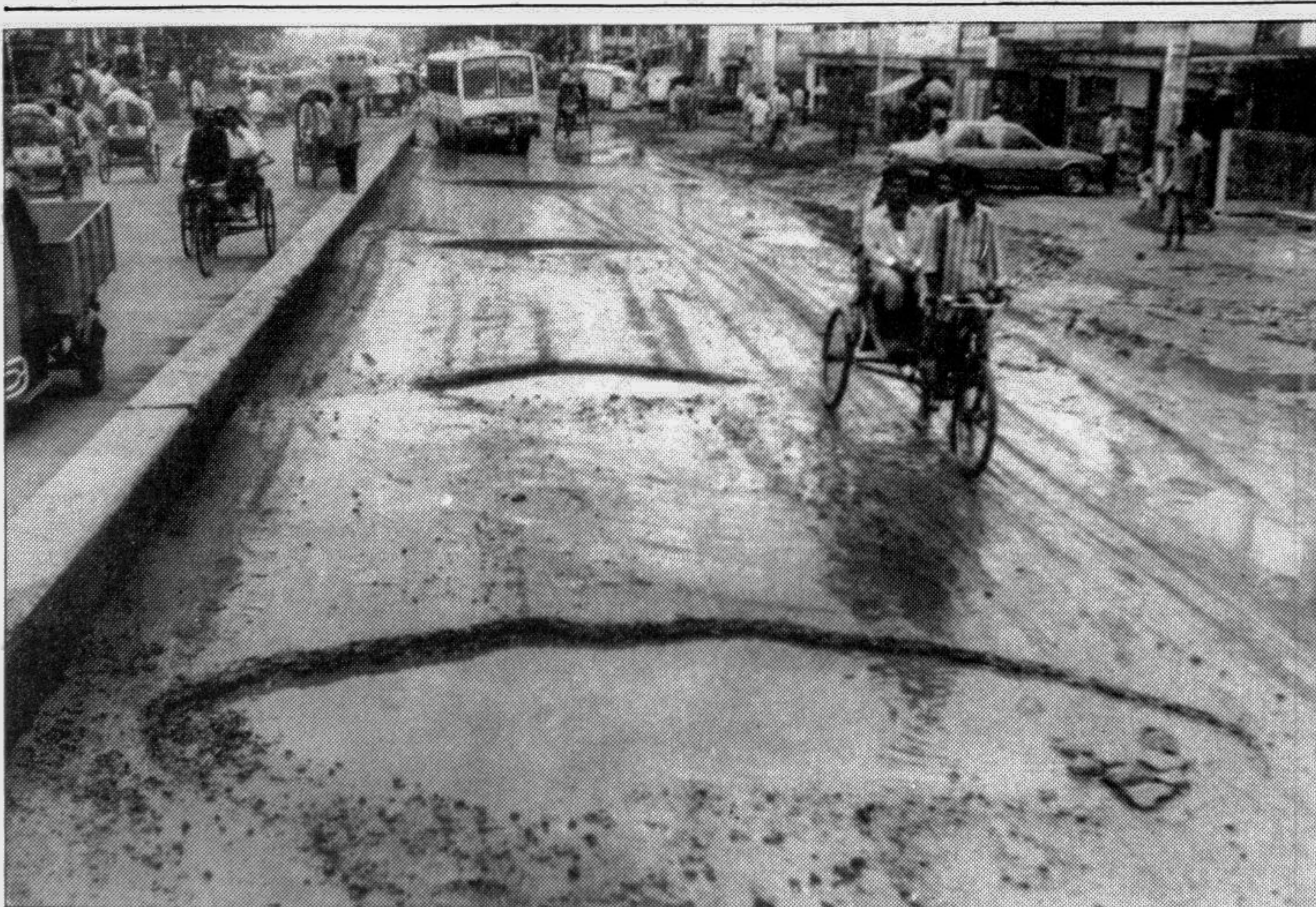
Big potholes have developed on the Bishwa Road near Maddhy Badda in the city due to incessant rains that continued for few days. — Star photo
