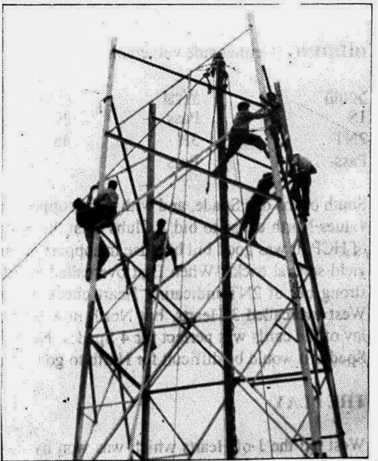
Workers disassembling one of the four floodlight towers at the Dhaka Stadium yesterday. These towers will be replaced by new ones to facilitate the ensuing ICC knockout one-day cricket tournament involving the nine Test-playing nations in October and November. — Star photo
