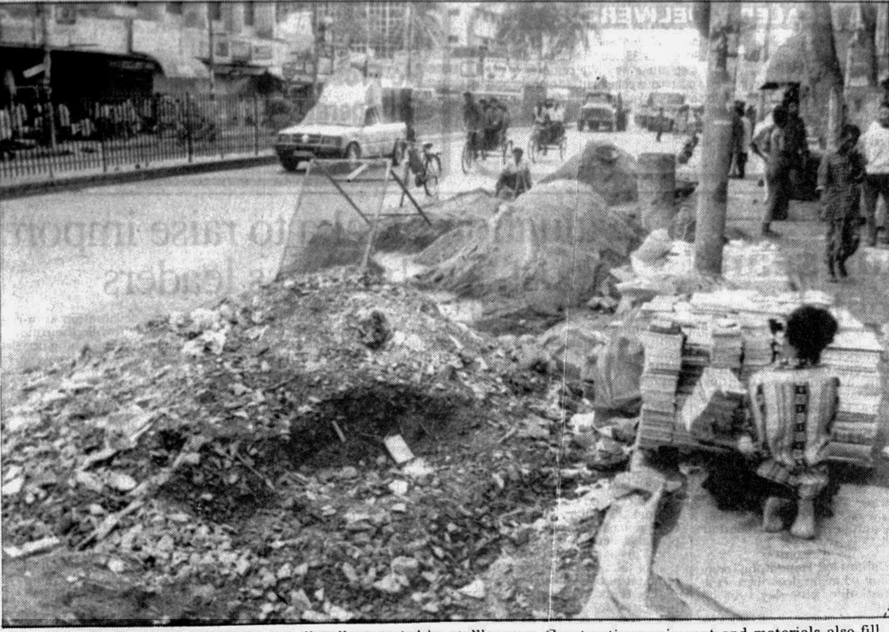
The footpaths in Baitul Mukarram are illegally occupied by stallkeepers. Construction equipment and materials also fill these sidewalks. -Star photo
