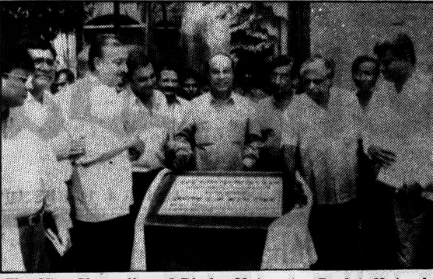
The Vice-Chancellor of Dhaka University Prof A K Azad Chowdhury laid the foundation stone of a new building of the Geology Department at the Curzon Hall premises yesterday.
