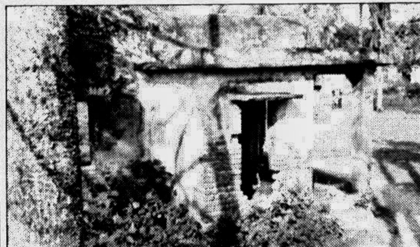
JHENIDAH: Abandoned Patwari quarters of Bangladesh Water Development Board (BWDB) situated at Bhalki in Harinakundu police station are being ruined due to indifference of the authorities concerned. — Star photo
