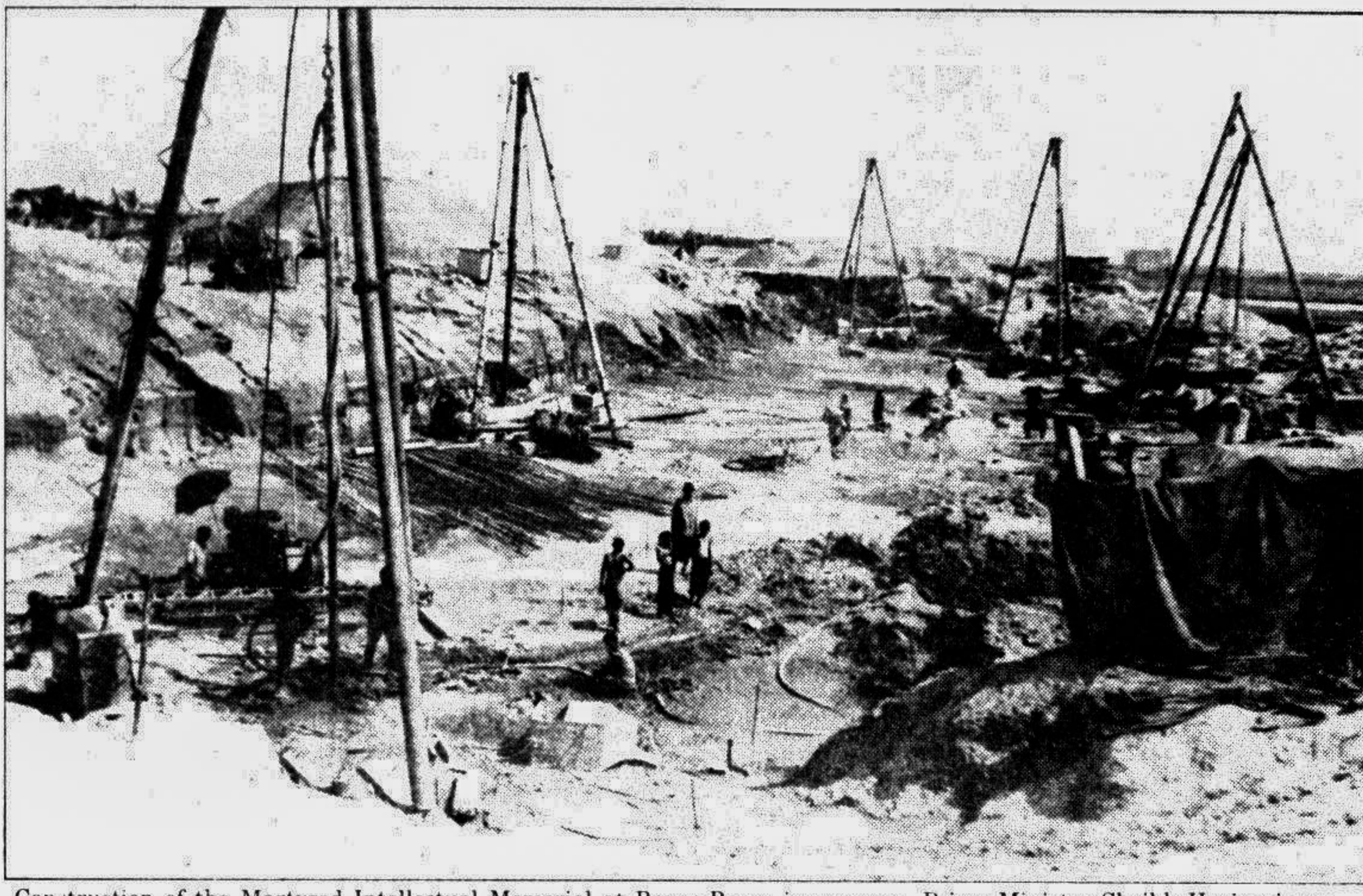
Construction of the Martyred Intellectual Memorial at Rayer Bazar in progress. Prime Minister Sheikh Hasina is expected to inaugurate it following completion of construction work by December 14, '98. — Star photo by Anisur Rahman
