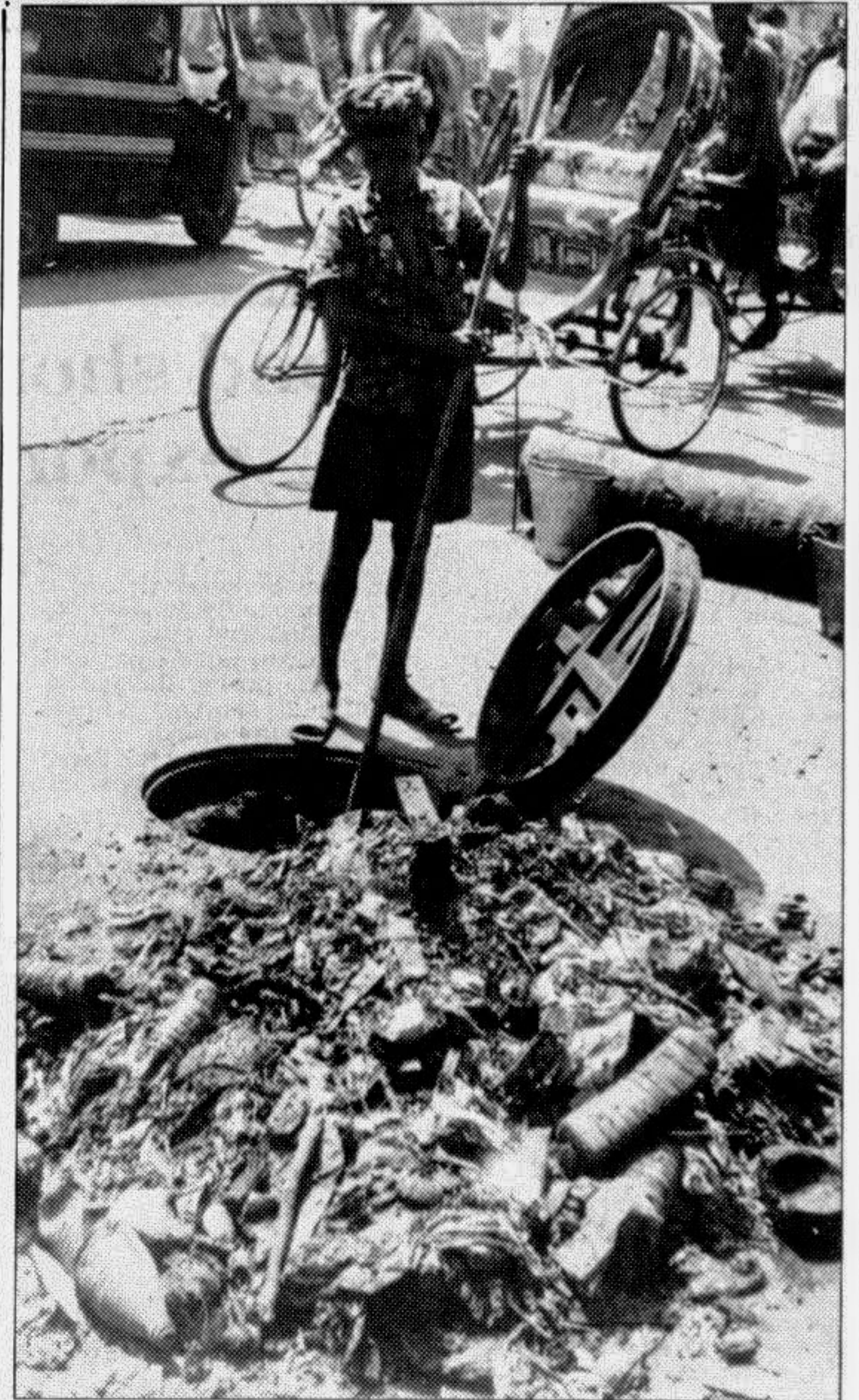
A street urchin giving Dhaka WASA a hand cleaning a sewerage line in the city. Most sewerage lines contain unwanted solid wastes, including polythene bags, plastic bottles and, other household refuse. The lines remain nearly clogged up round the year. — Star photo
