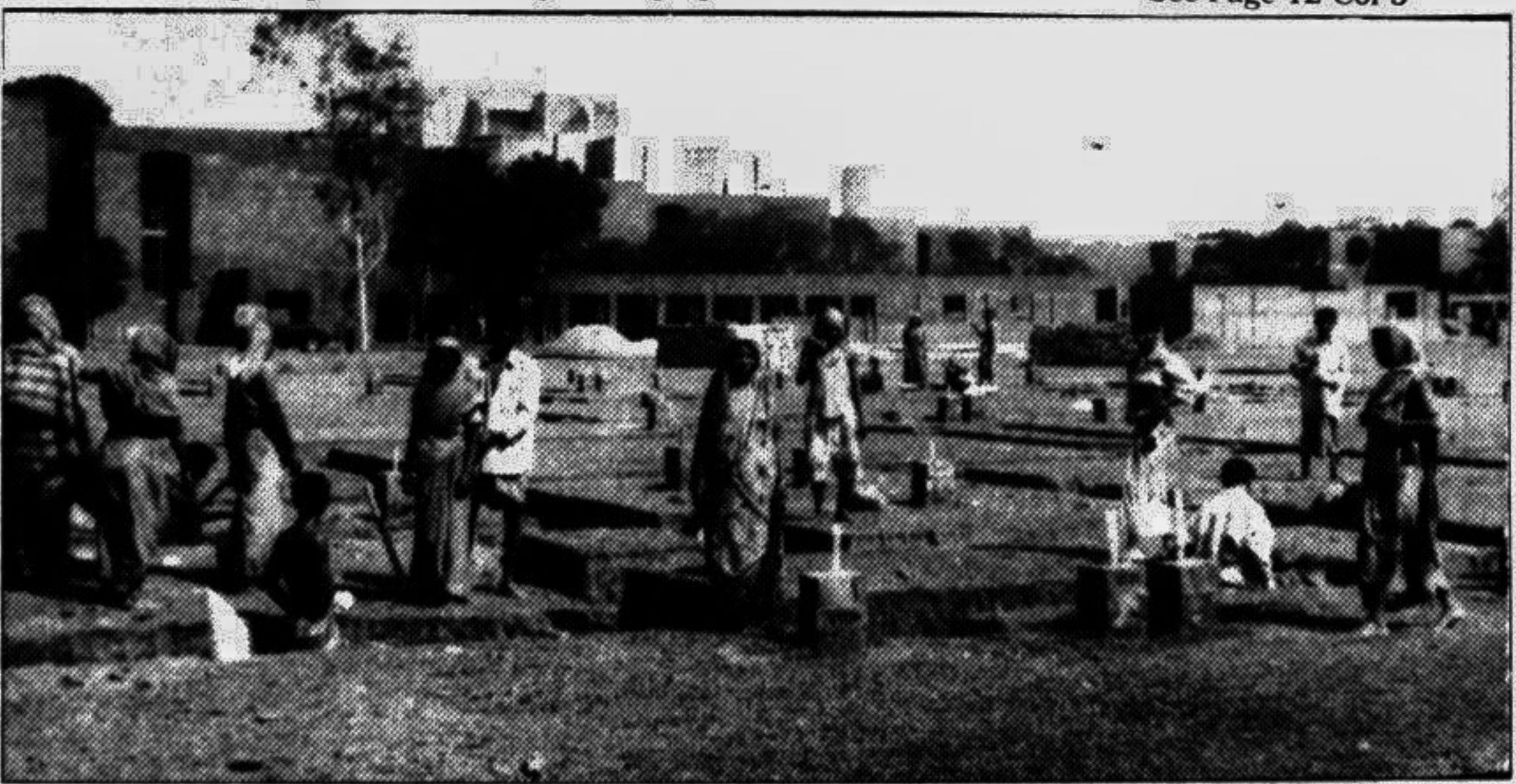
Construction work of official residences for the Speaker and the Deputy Speaker is going on in the Sangsad Bhaban area. — Star photo
