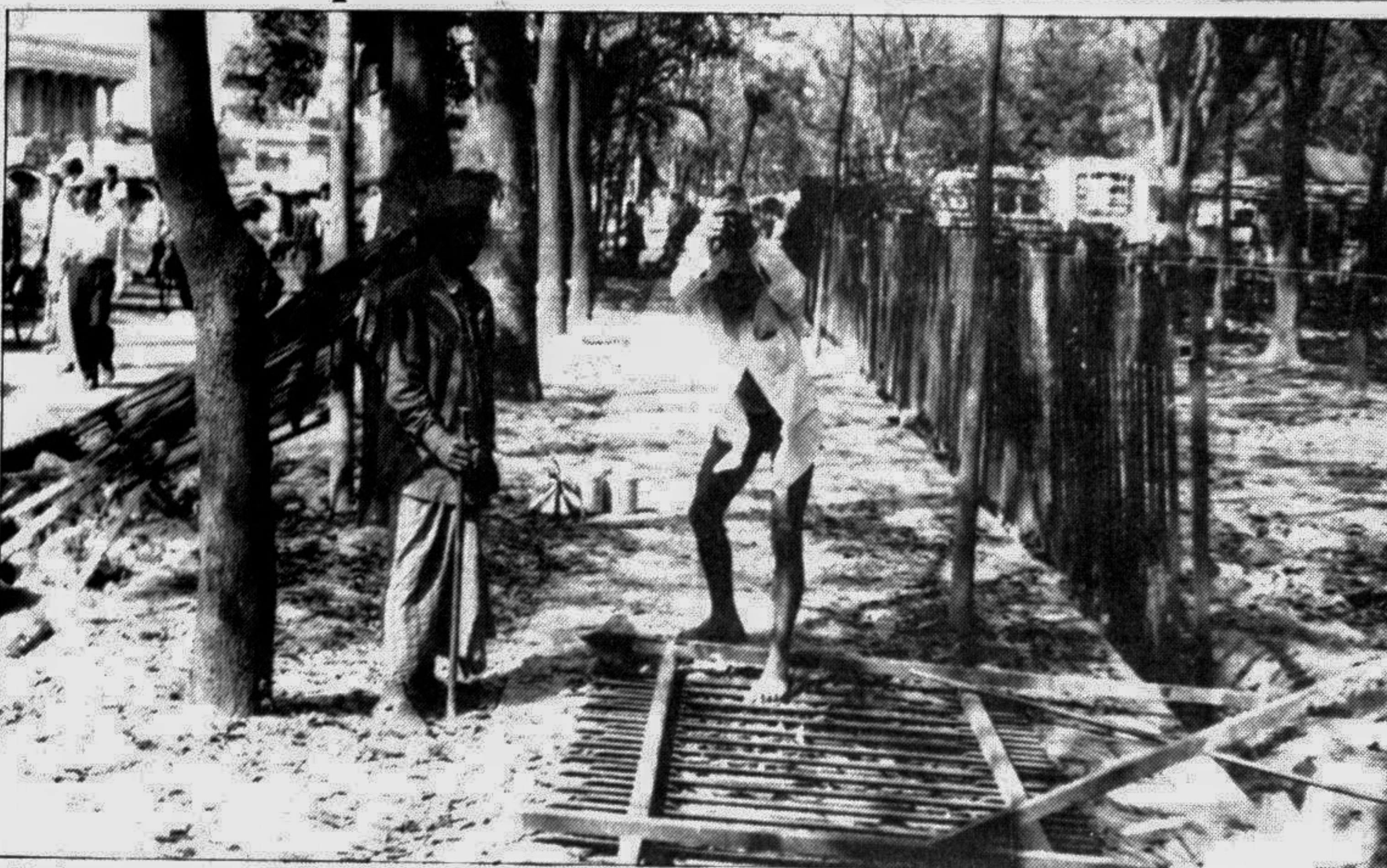
Workers removing iron railings from the south side of Osmani Uddayan for expansion of the road in front of Nagar Bhaban. —Star photo
