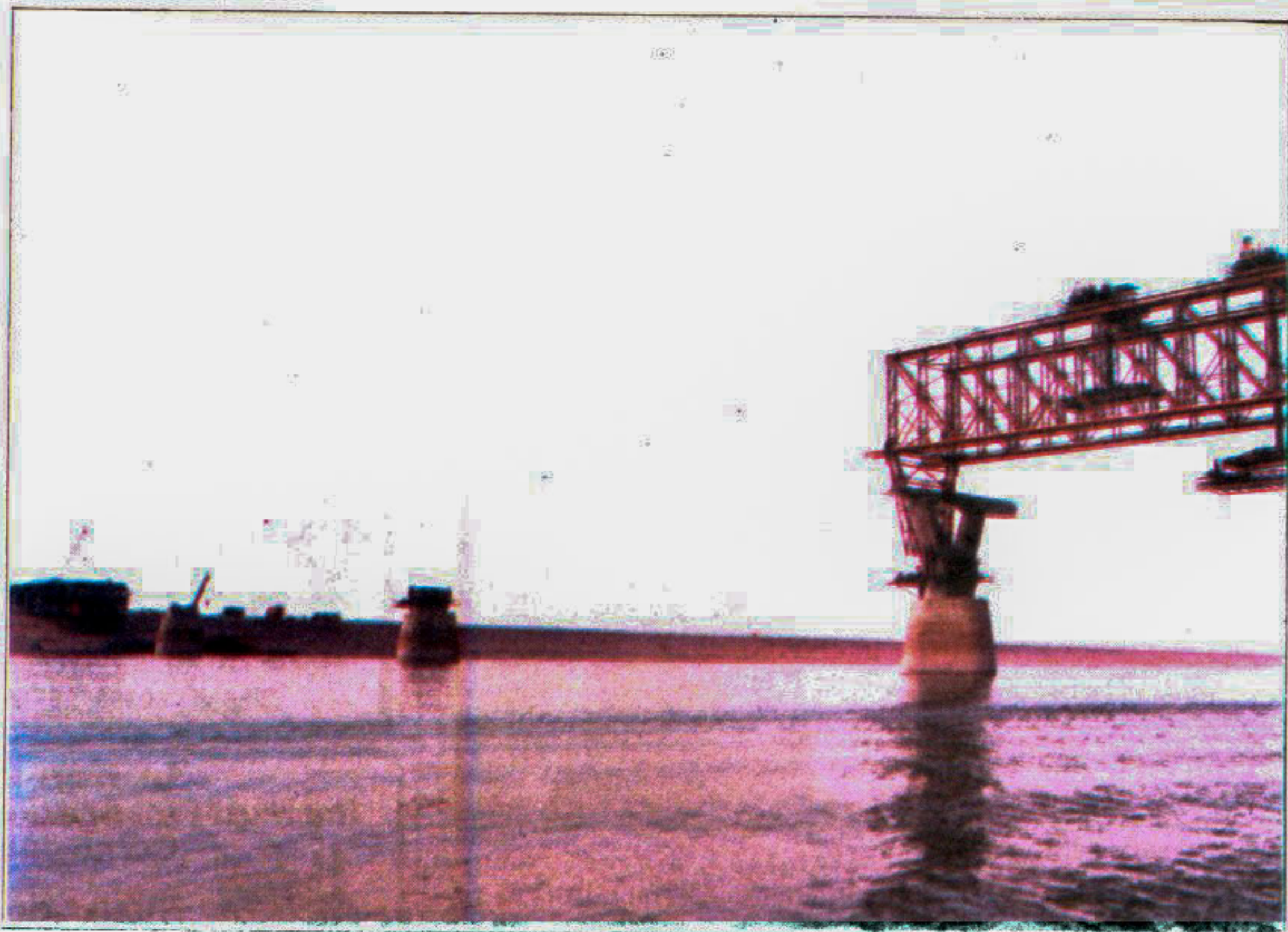
ONLY-THREE SPANS LEFT: The bridge on the Jamuna is fast nearing completion. It is scheduled to be opened to traffic on June 23 this year. The billion-dollar bridge is 4.8 km long and the longest in the country.
