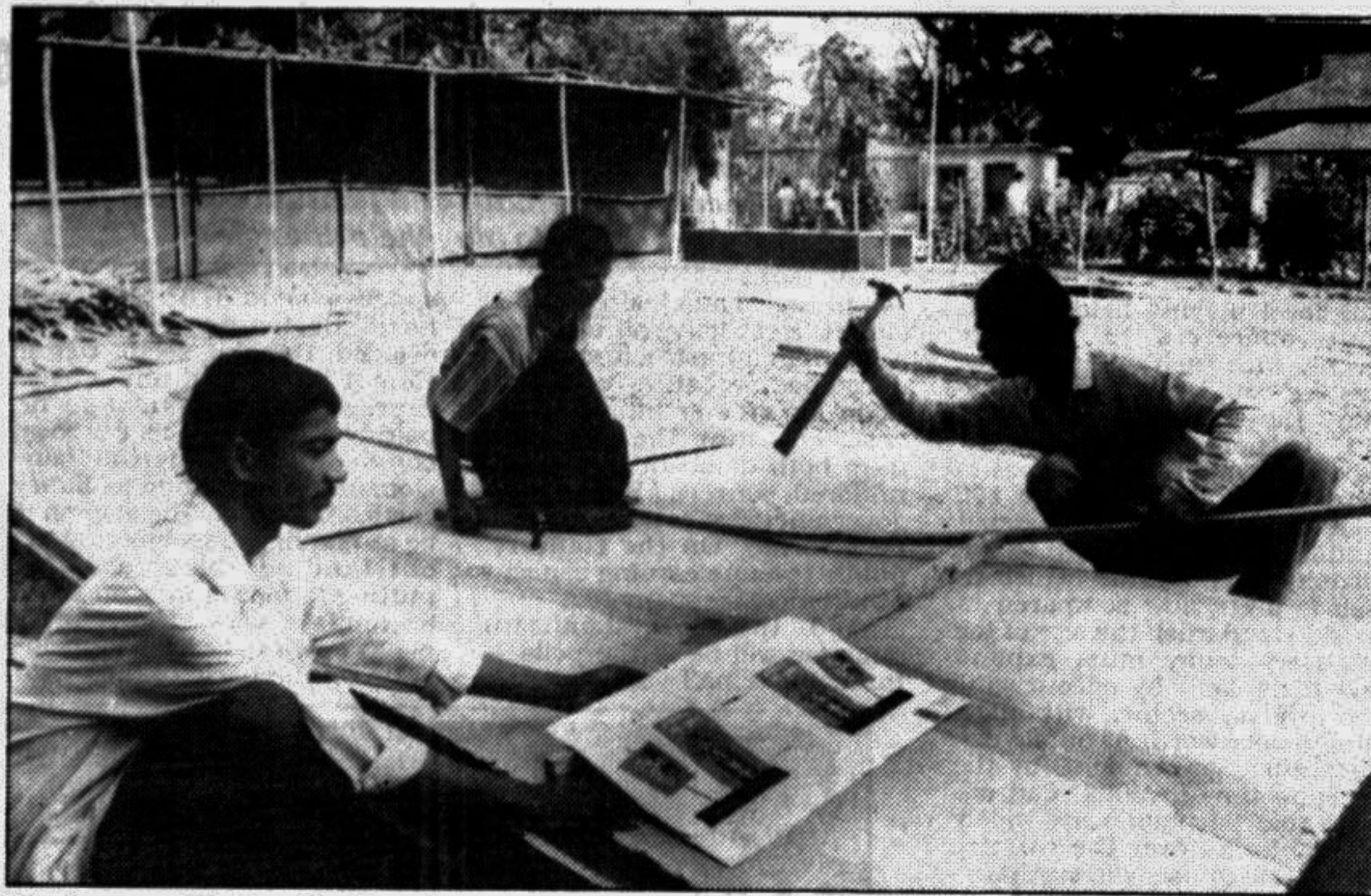
Work on stalls for the Bangla Academy Boi Mela '98, which begins from Feb 7, is going on in full swing on the Academy premises in the city. —Star photo
