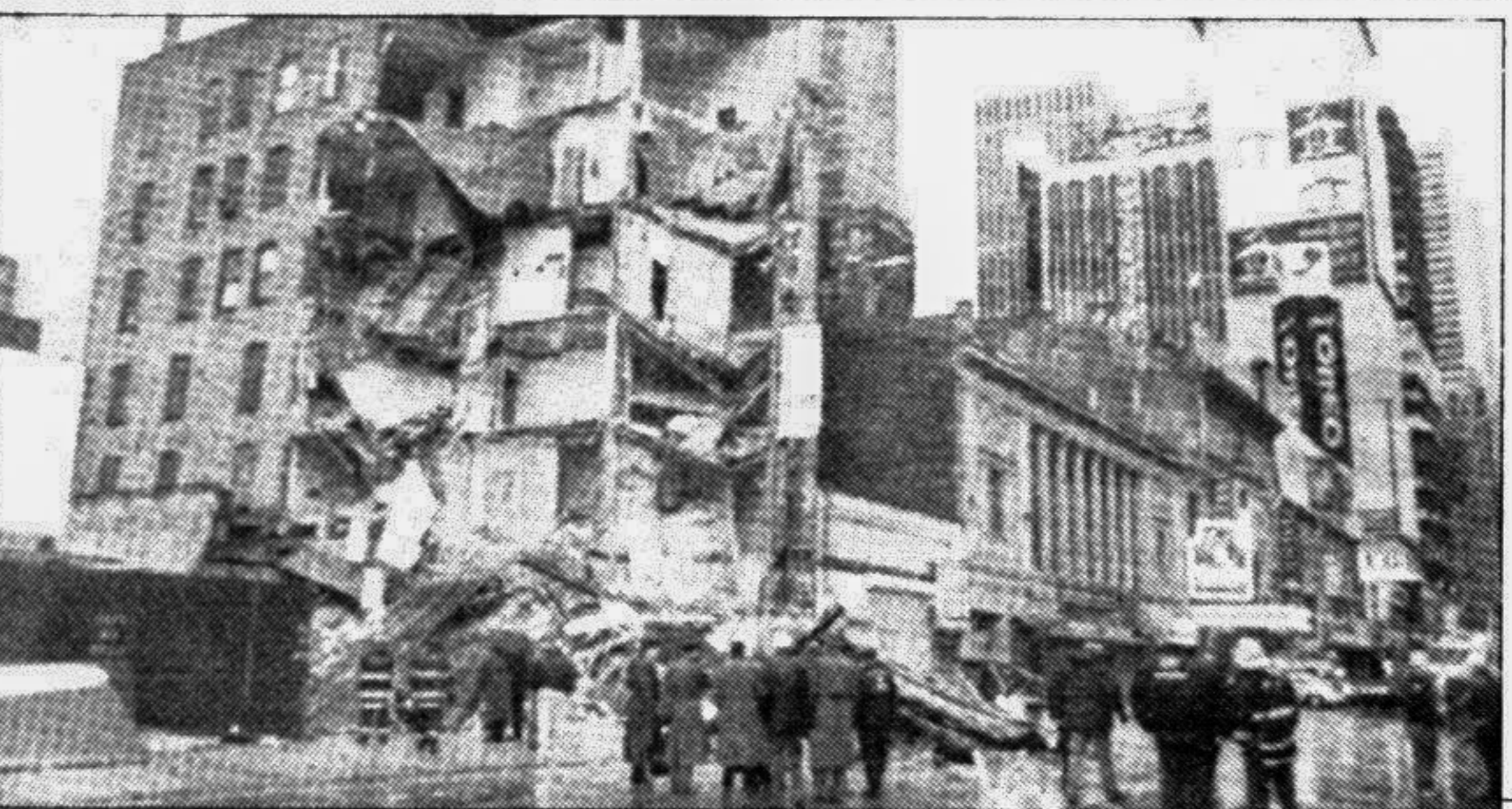
Officials look at the six-story building on 42nd Street that collapsed early Tuesday morning in New York. The building, holding balloons and other items for the annual New Year's Eve celebration, was unoccupied at the time of the collapse and had been slated for demolition in the spring. No one was injured in the collapse, said Fire Department spokesman Frank Zitaglio. — AP/UNB photo
