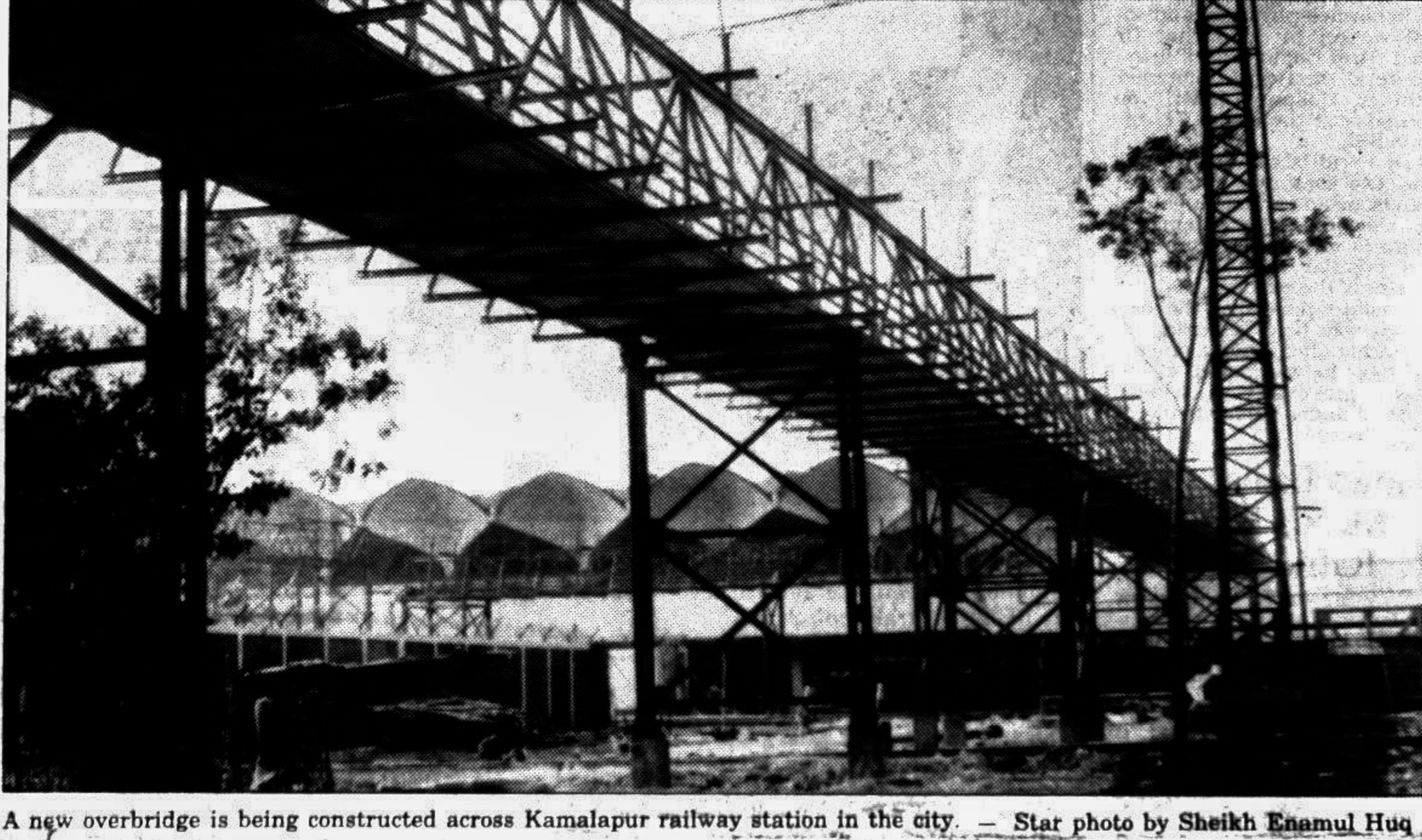
A new overbridge is being constructed across Kamalapur railway station in the city. — Star photo by Sheikh Enamul Haq
