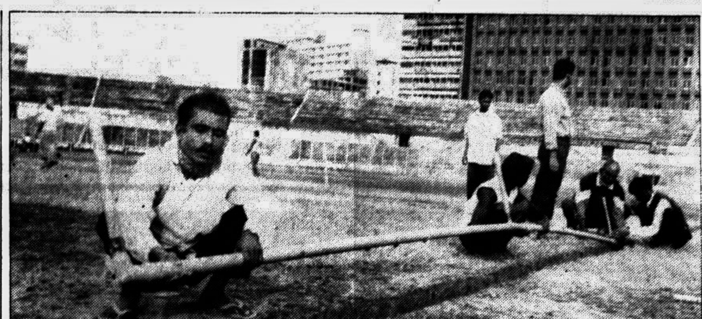
PREPARING FOR THE BIG EVENT: With the Independence Cup drawing nearer, grounds-man at the Dhaka Stadium are seen busy with installing the pipeline down the pitch to accommodate the stumpvision camera for the WorldTel. The famous electronic media who will cover the three-nation tourney involving India, Pakistan and hosts Bangladesh.
