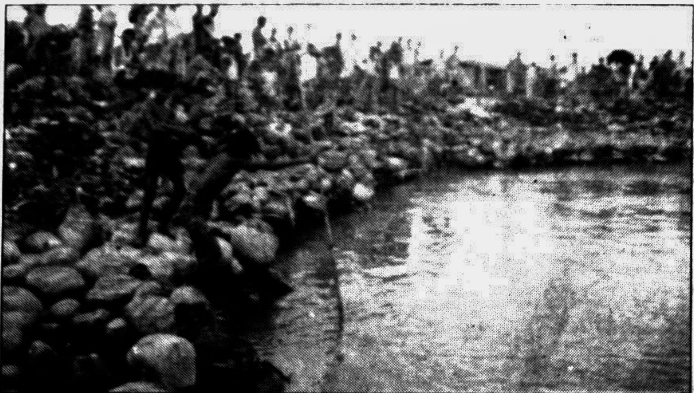
CHANDPUR: Boulders being eroded from the town protection embankment by the river Meghna in Chandpur town. — Sun photo
