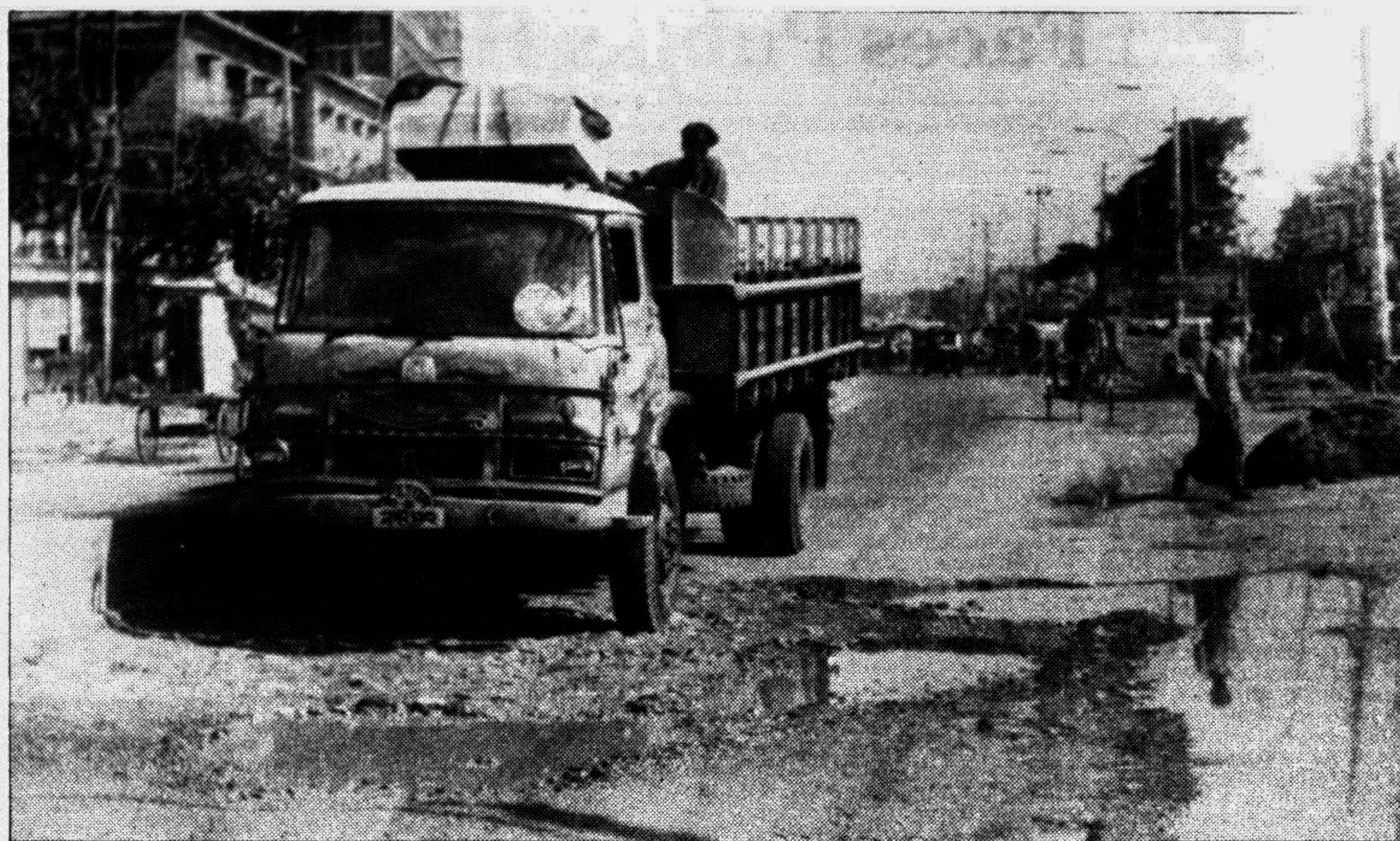
Potholes in the busy road at Bishwa Road (in Maddhya Badda) have been causing inconvenience to the movement of vehicles and the pedestrian for a long time. — Star photo
