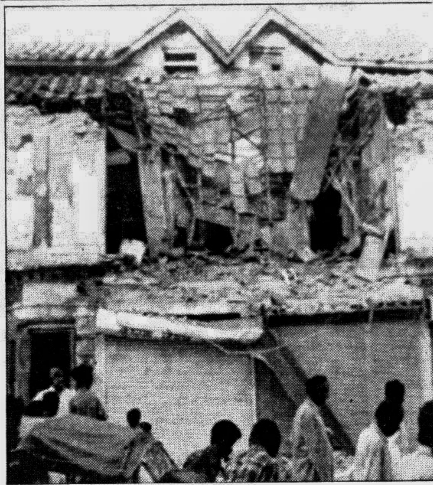
A house damaged by earthquake that hit Jabalpur in India on Thursday. — AFP UNB photo
