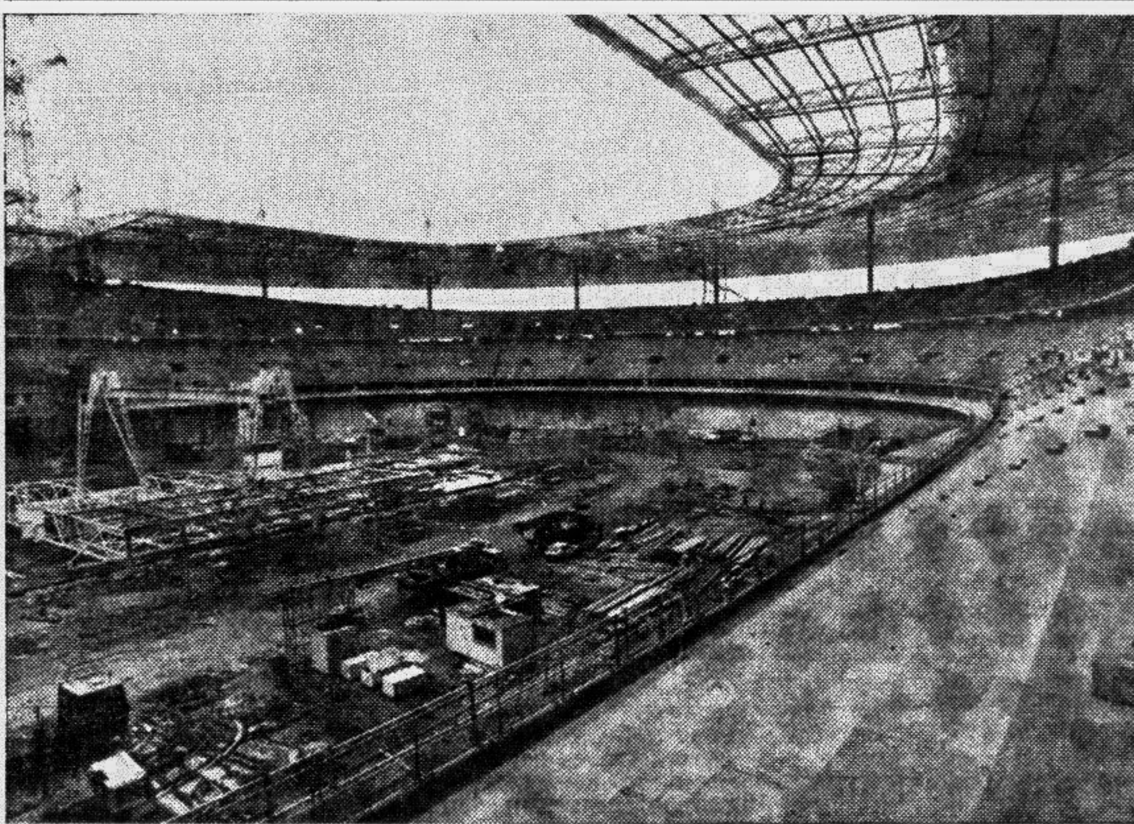
AFP filmed this view of an under construction stadium at Saint-Denis in northern Paris on May 20. Works are going in full swing at this 1998 World Cup venue.
