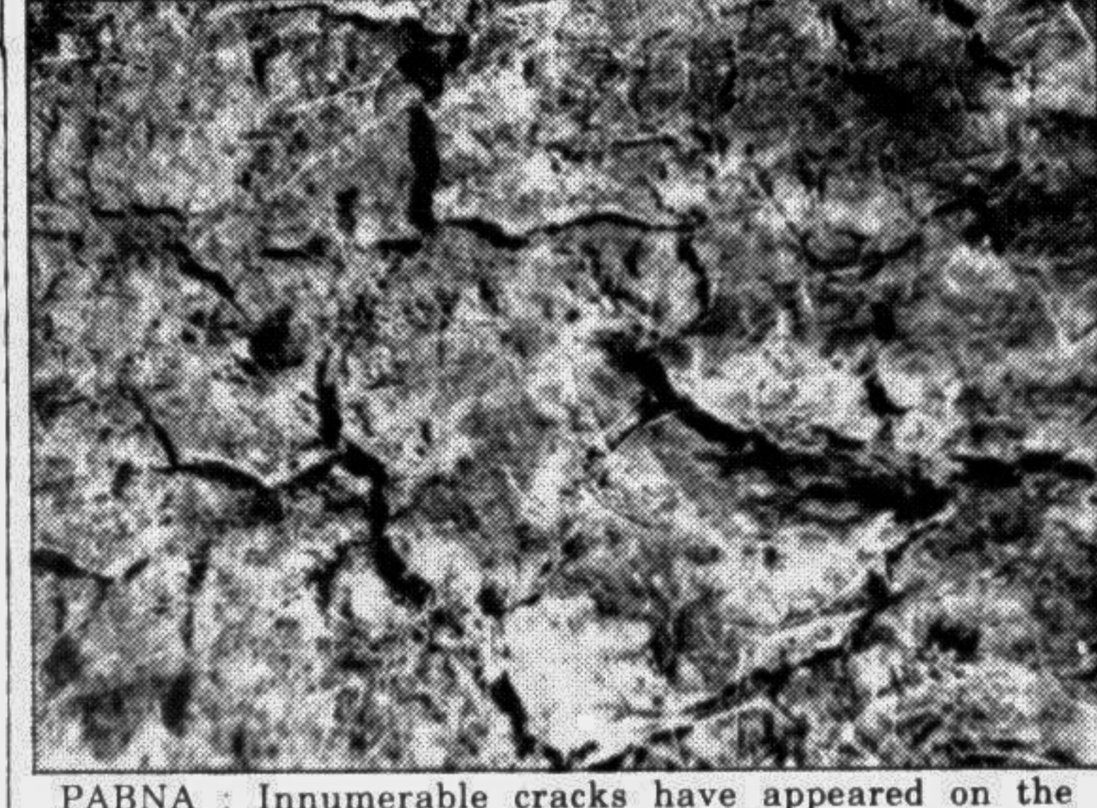
PABNA: Innumerable cracks have appeared on the cultivable land in a village under Debottar union of Atgharia thana in the district — Star photo
