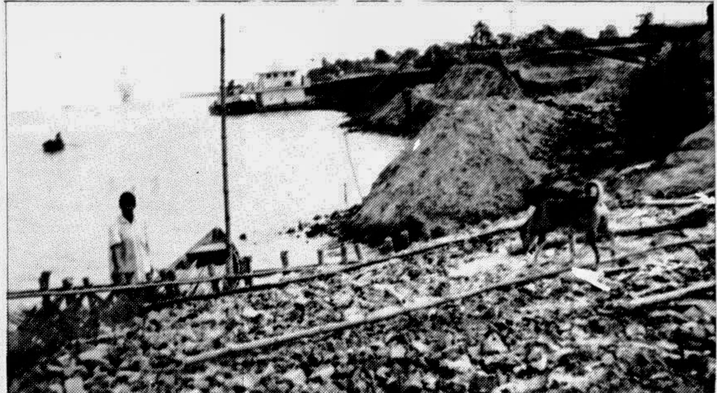
PABNA: Despite temporary steps to check serious erosion of the river Jamuna near Raghunathpur, the temporary approach road from Nagarbari to Natakhola ferry ghat has been facing a serious threat of damage.
