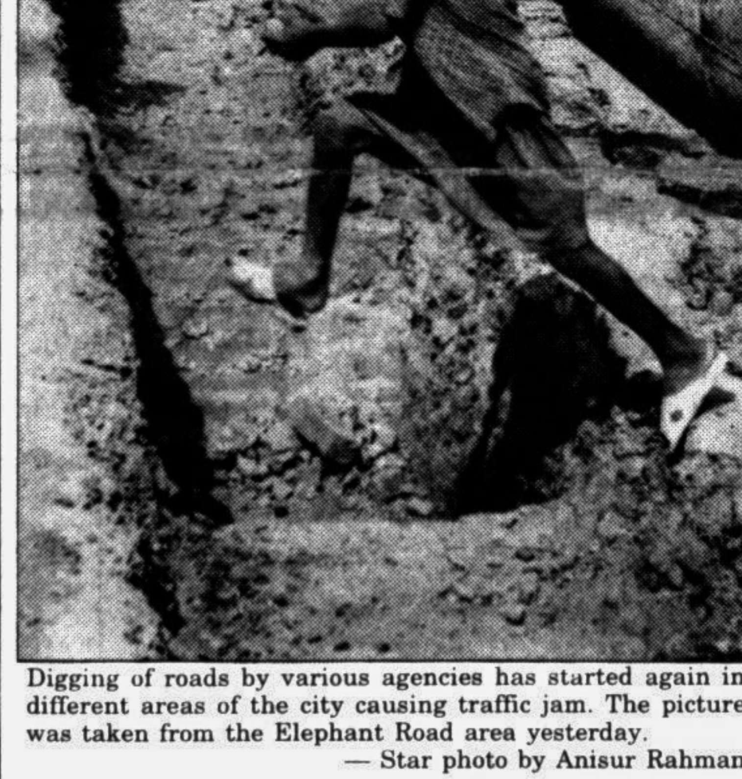
Digging of roads by various agencies has started again in different areas of the city causing traffic jam. The picture was taken from the Elephant Road area yesterday.
