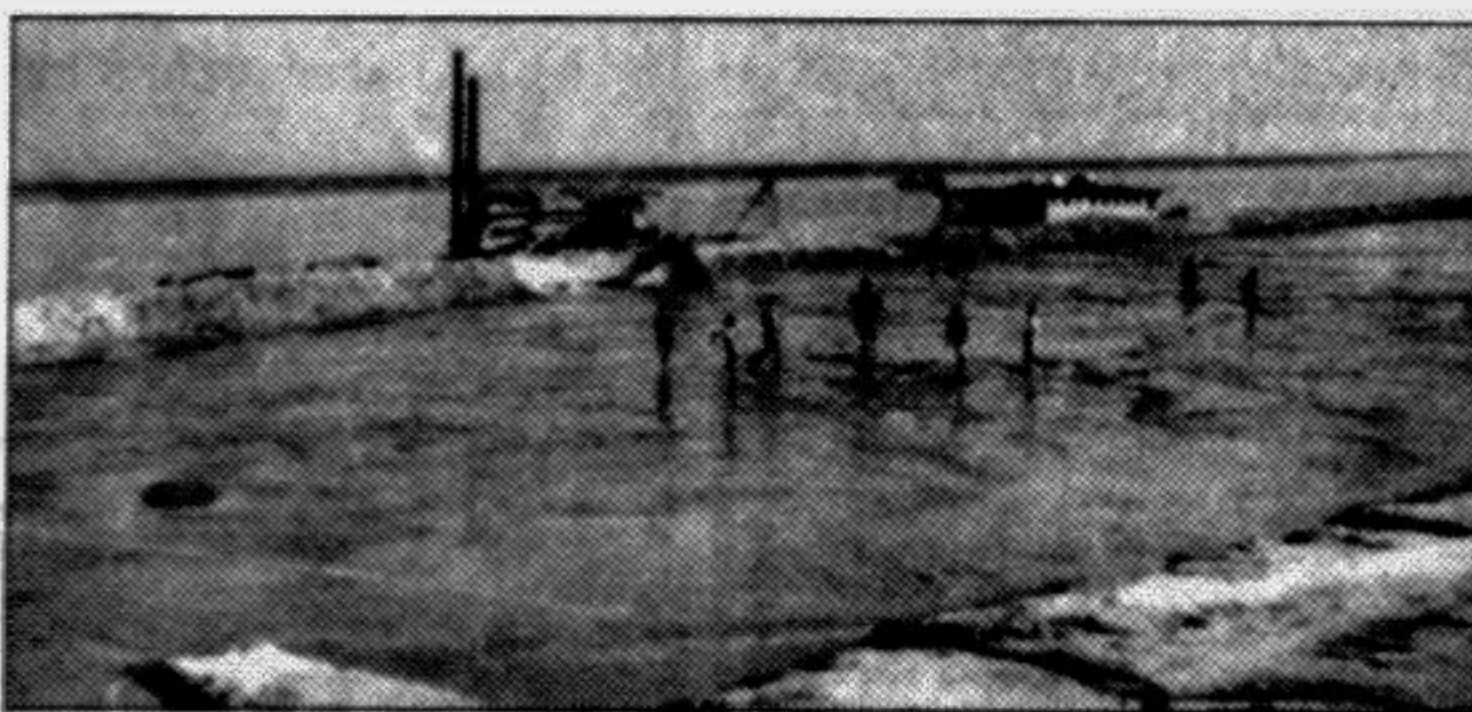
PABNA: Dredging started by the BIWTC at the downstream of Nagorebari ghat for keeping the ghat operational for barges and cargo vessels. — Star photo
