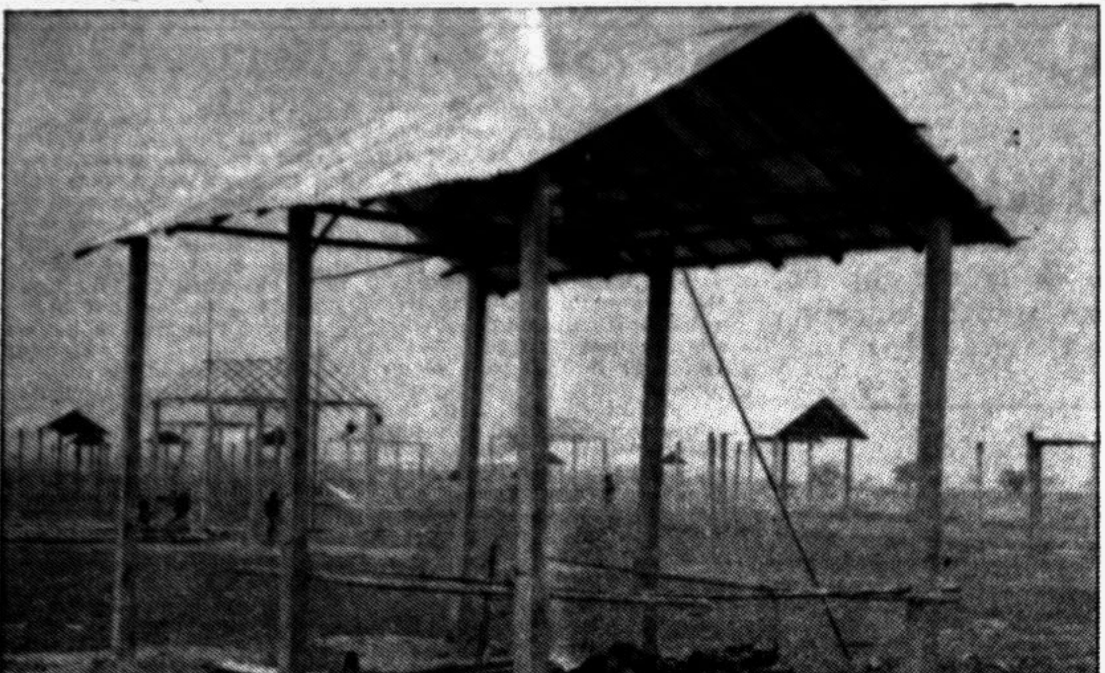
RAJSHAHI: Tinsheds houses are being set up on the charlands of the Padma for landless people under Charland Development Project taken up by the Ministry of Land. This photograph was taken from Char Taranagar under Harijan union of Poba thana in the district. Rehabilitation of landless, homeless people under the project has already begun in the neighbouring areas. — Star photo by Abdul Wadood
